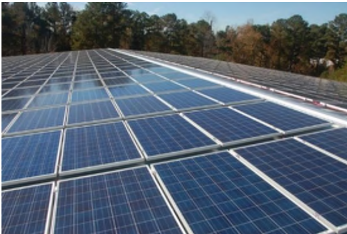
Figure 3: Rooftop Solar with Minimal Spacing
