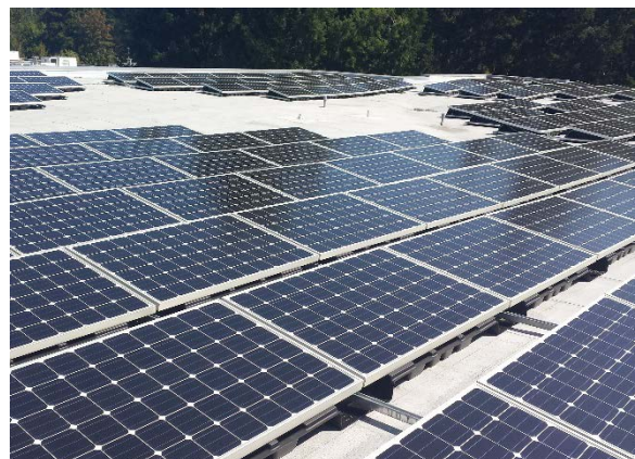
Photovoltaics used for Bellevue College solar project
