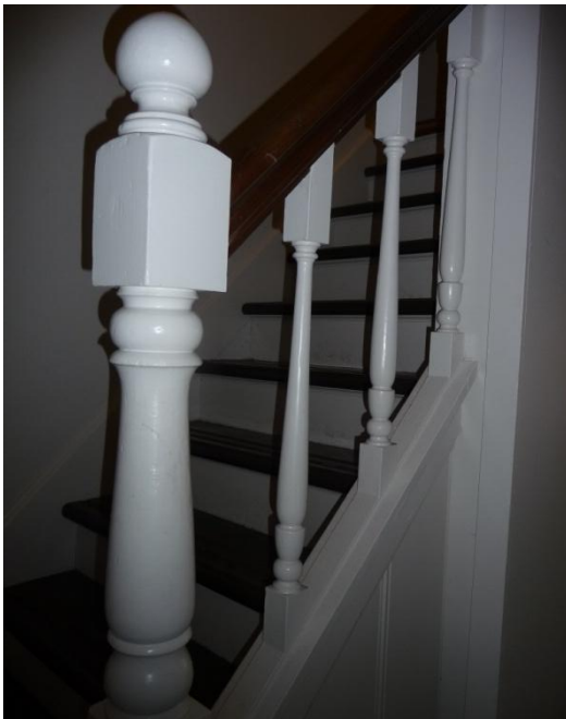
North Unit Stair Rail
