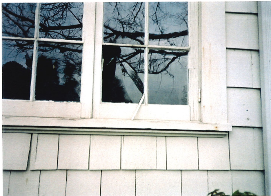
B: ASBESTOS-CONTAINING WINDOW PUTTY; EXTERIOR WINDOW.
