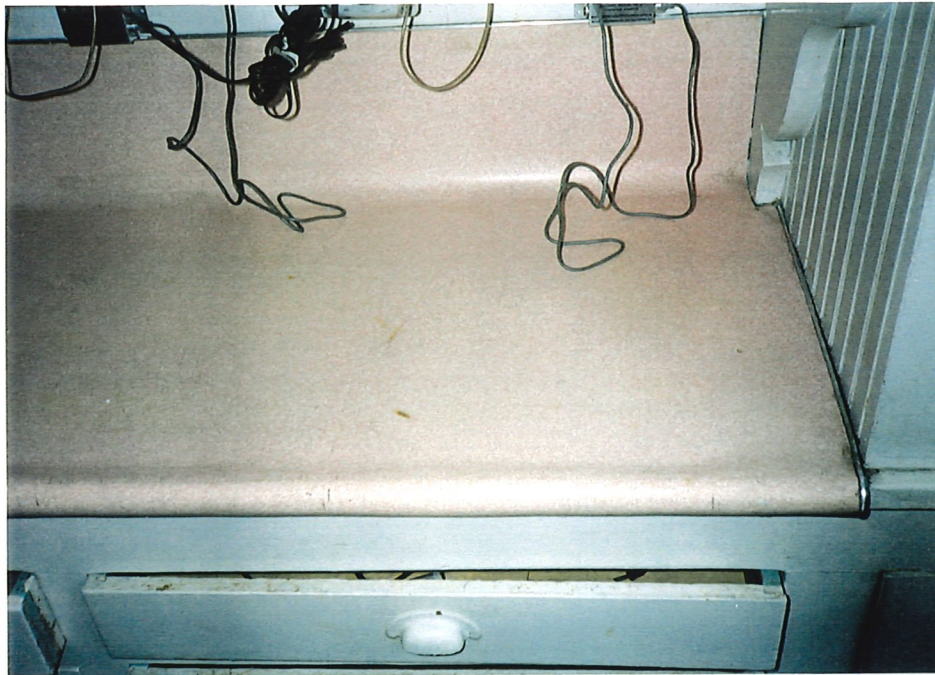
A: ASBESTOS-CONTAINING SHEET VINYL; KITCHEN COUNTER.
