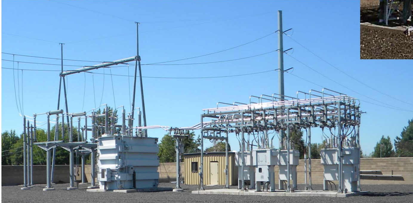
Nelson Road Substation
