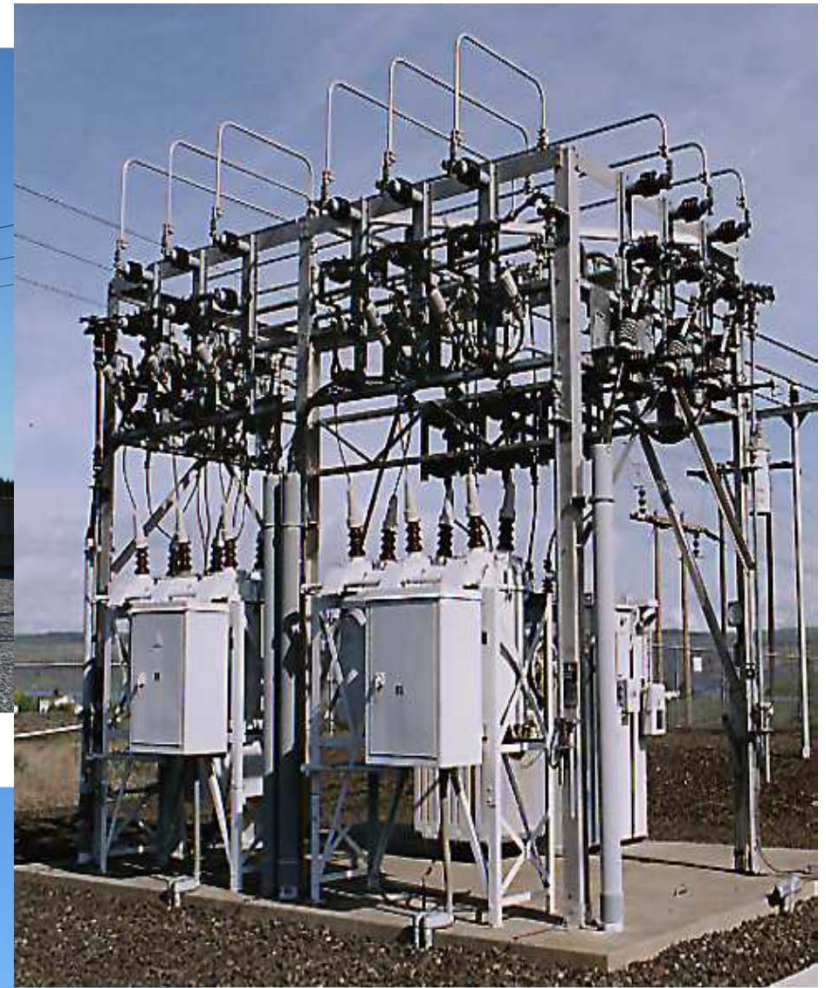
Coulee City Substation
