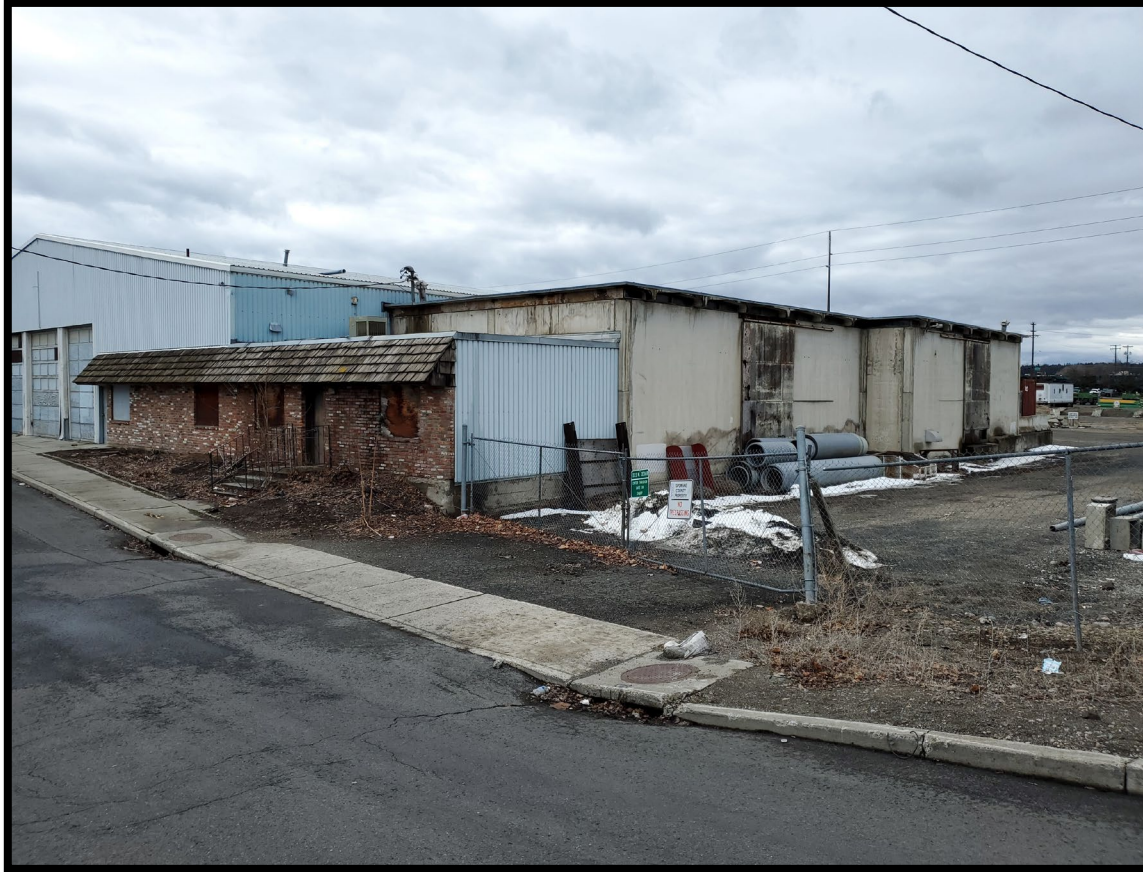
Heavy water damage and structural damage to exterior of all buildings
