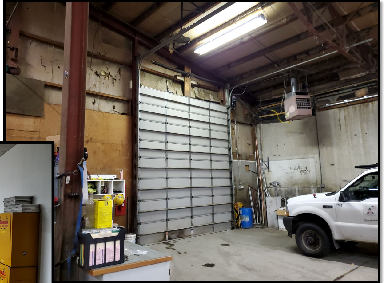
Water damage and structural damage to walls
