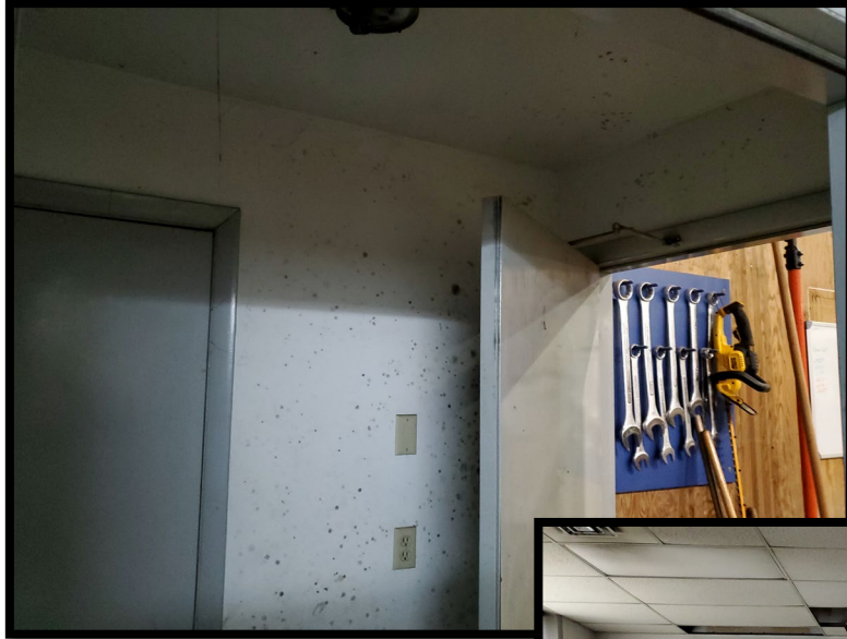
Black mold on walls
