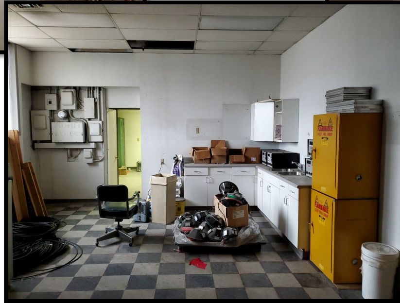
Water damage and structural damage to walls, floors, and ceiling
