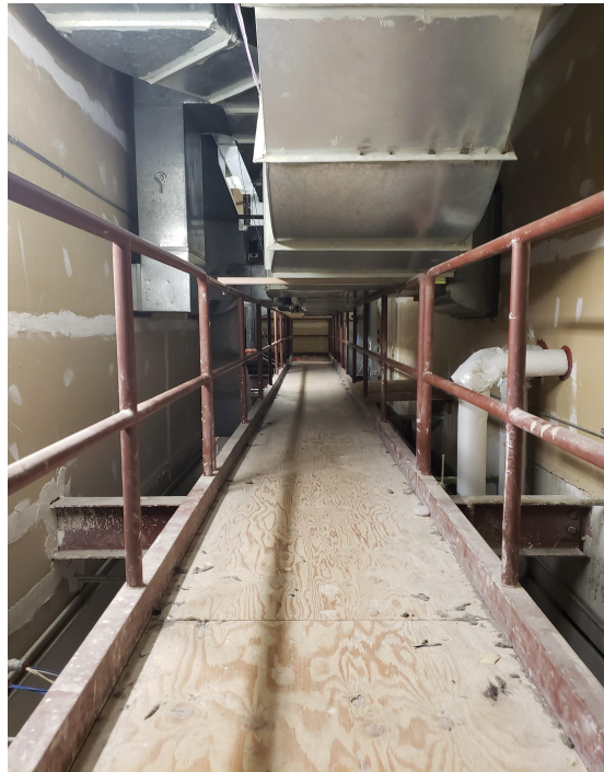
MTH plenum catwalks (1989)
