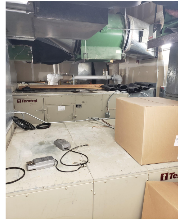
MTH air handling units (rebuilt 2017)
