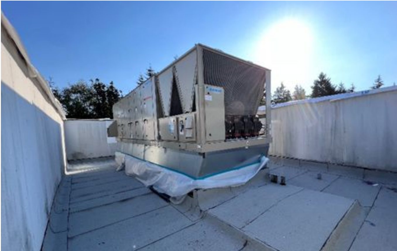
ESD Educational Services Center replaced air handler / chiller
