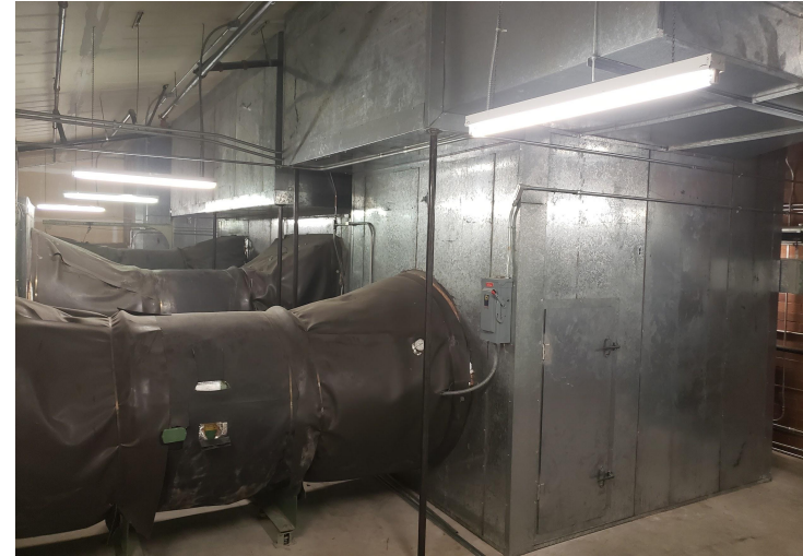
MTH supply fans, return fans, & filter banks (1989)
