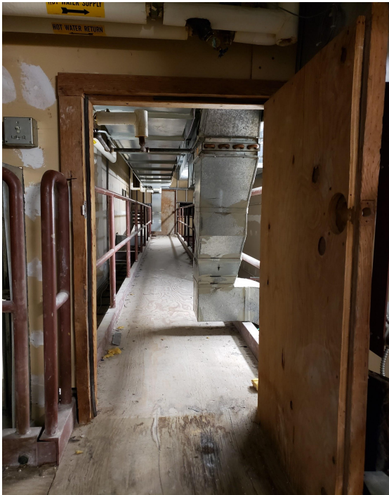
MTH plenum catwalks (1989)
