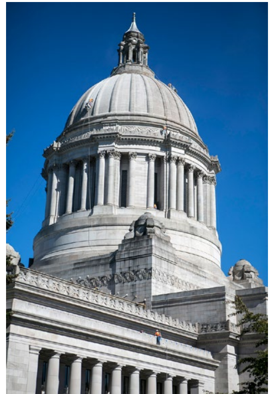
Legislative Building roofing and masonry repairs for the State of Washington in Olympia.
