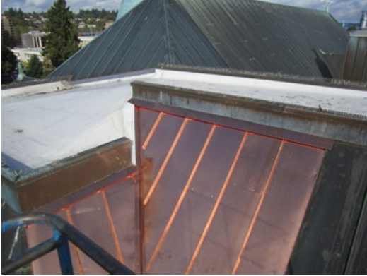
SHKS designed limited roof repairs performed as part of the 2015 Old Capitol Building Exterior Restoration project.
