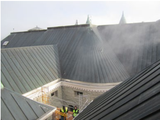
Investigations of masonry cladding and drainage conditions at the Old Capitol Building.
