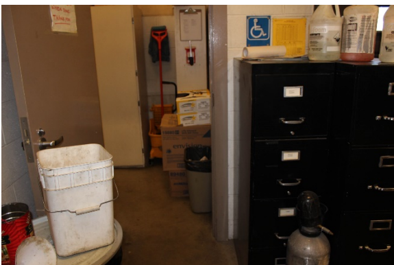
Doorway into bathroom is not ADA accessible
