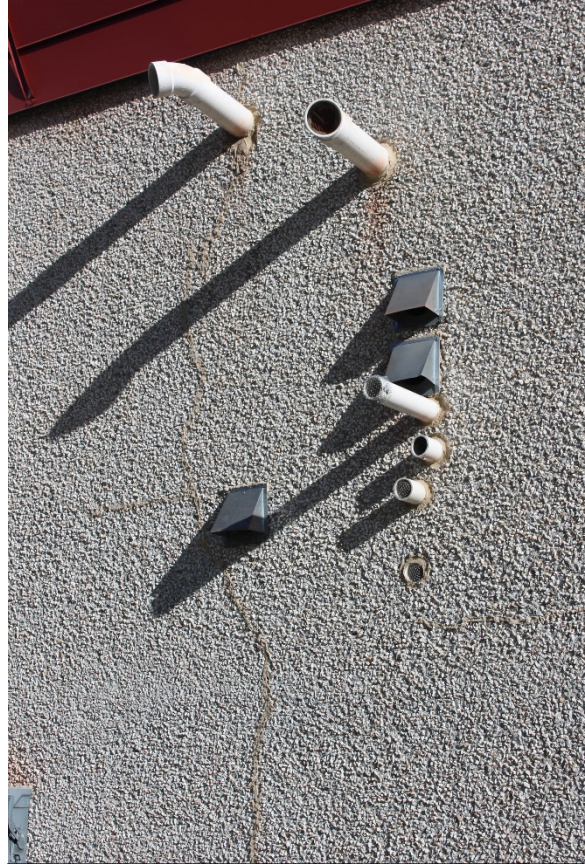
Cracks up the side of the walls surround the building
