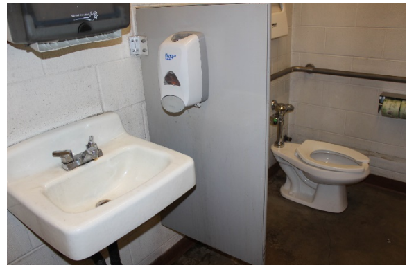
The only bathroom in the building, not ADA accessible
