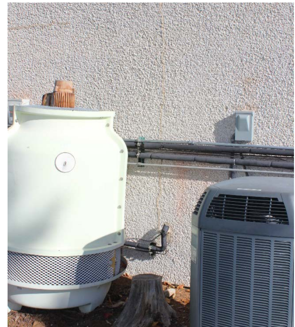
Cracks on the building's exterior align with locations of old stumps
