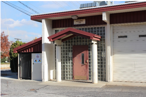
Building entrance is surrounded by glass blocks and gases are stored to the left of the entrance
