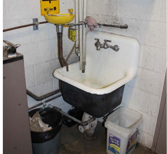
Antique sink that services the building
