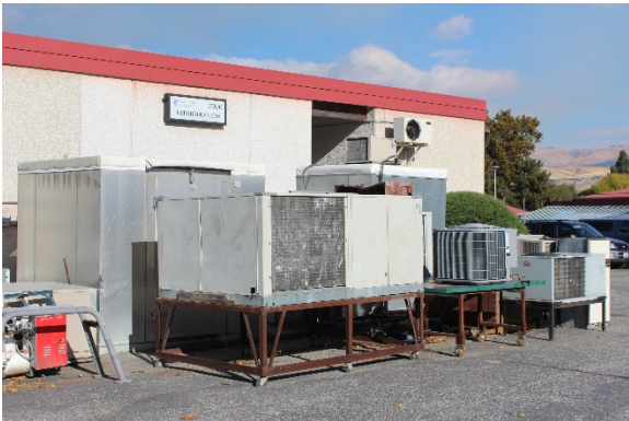
HVAC units are stored outside of building due to lack of storage
