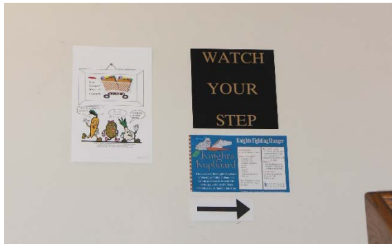
Signs stating, 'Watch your step' are posted in the stairways leading up to the second floor. Stairs are uneven and chipped in places
