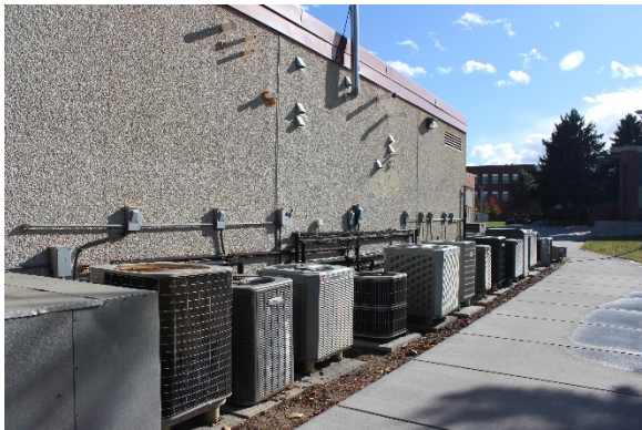
HVAC units line the exterior of the facility
