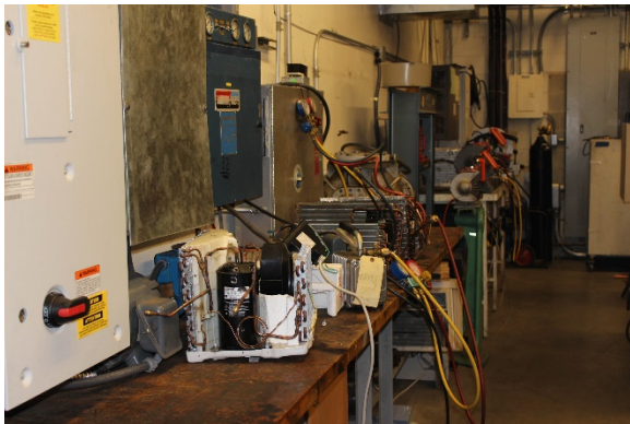
Workspaces lack storage and counter space
