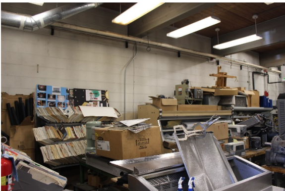
HVAC systems in the buildings were installed by students years ago
