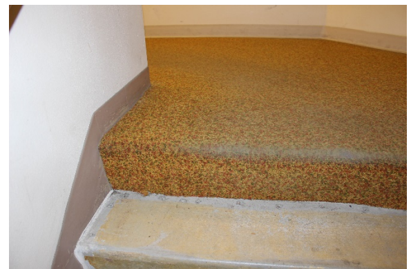
Carpeting in the stairway has been partially ripped up. Existing carpeting is stained.
