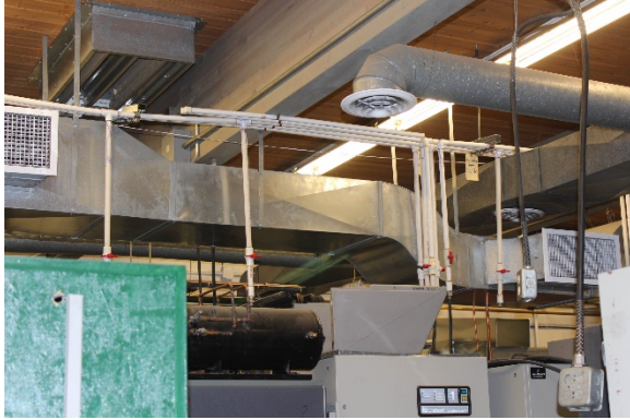
Units are packaged to the ceiling due to lack of storage space
