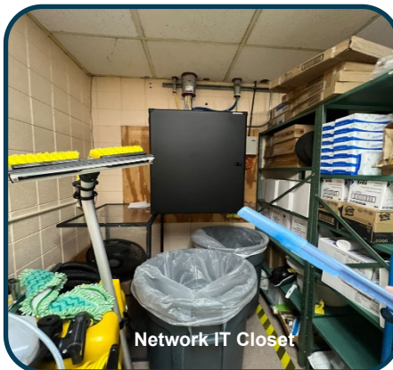
Domestic Water Main Service Entrance
