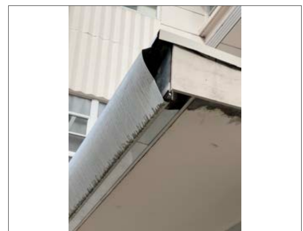
Frieze, aluminum showing a detail of the lower south facade canopy configuration.
