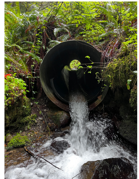
Existing Culvert with Temporary Repair
