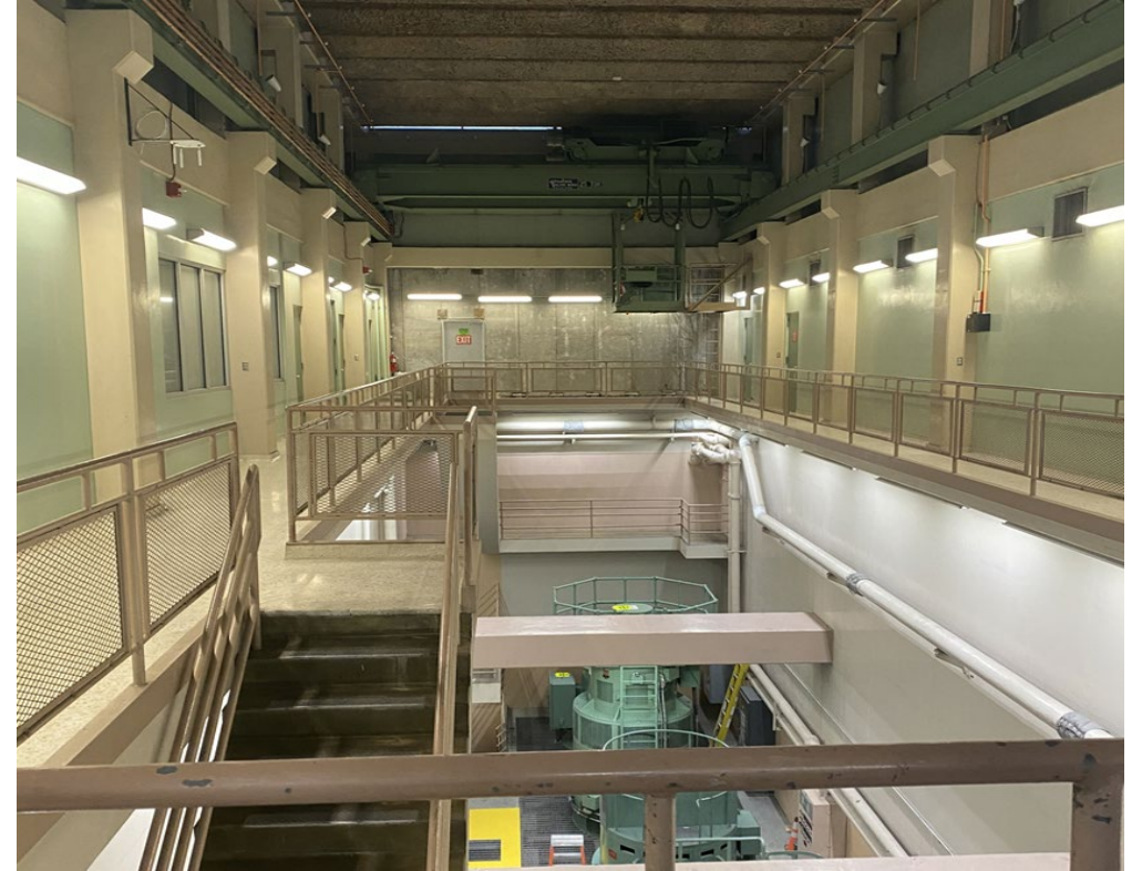
Pump Building – Crane Hall Gallery view
