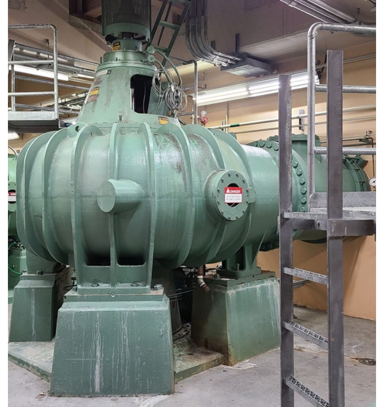
Raw sewage pumps
