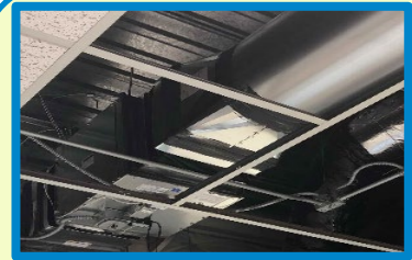
Pictured – HVAC Upgrade Tacoma Community College
