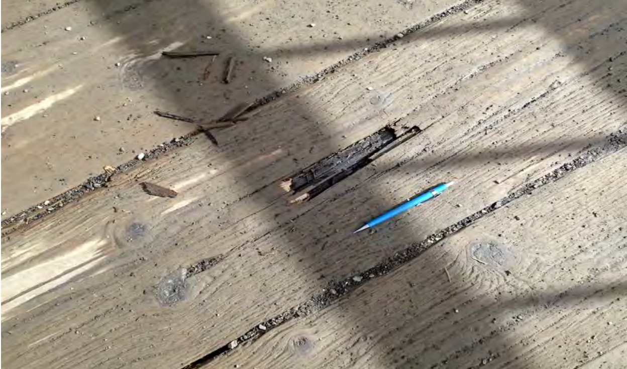
Photos 5 & 6 - Rotten Deck Boards-from above and below
