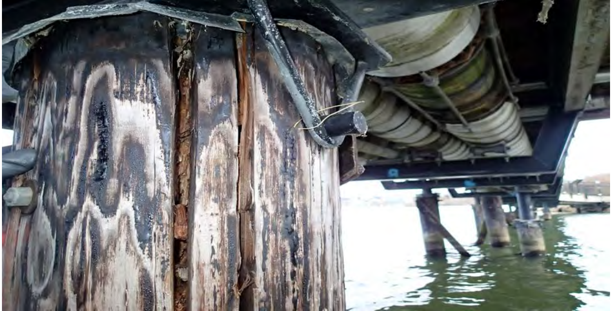
Photo 1 - Example of Rotten Pilings - Pile 7C is badly split with internal rot at the top
