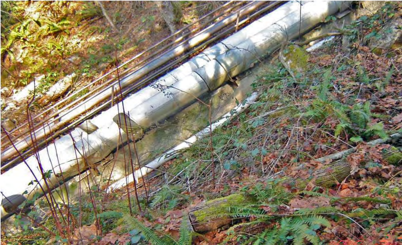
Damage to infrastructure, such utilities, roads etc.
