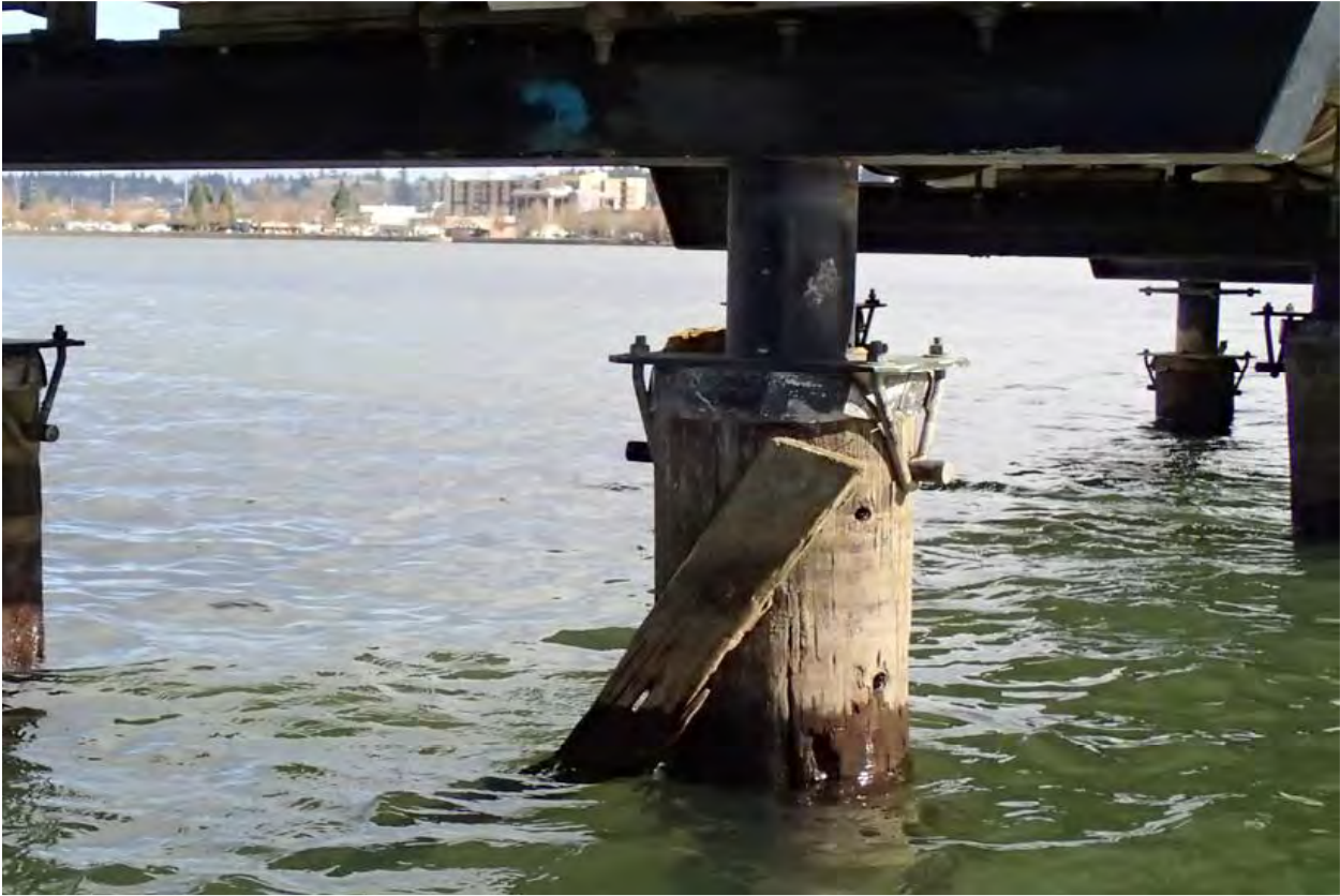
Photo 3 - Typical abandoned bolt holes in piling and section loss in bracing member
