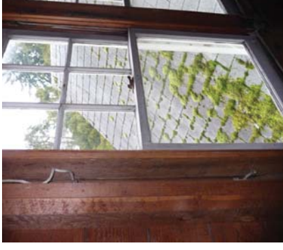
Broken sash chord
