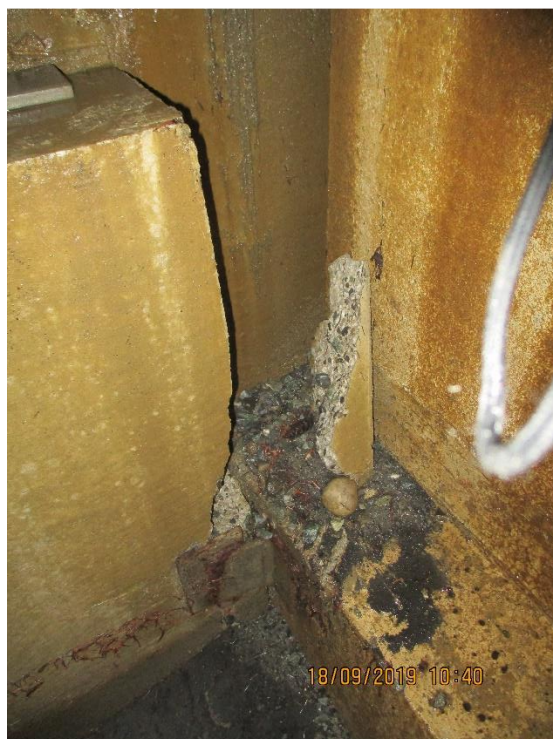
Photo 4- Spalling grade beam connection (typical condition)
