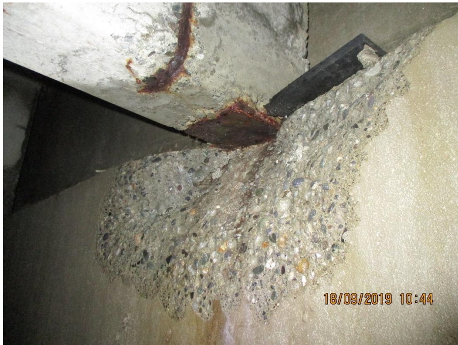
Photo 11 - Spalling of double-tee joist and its support (typical condition)
