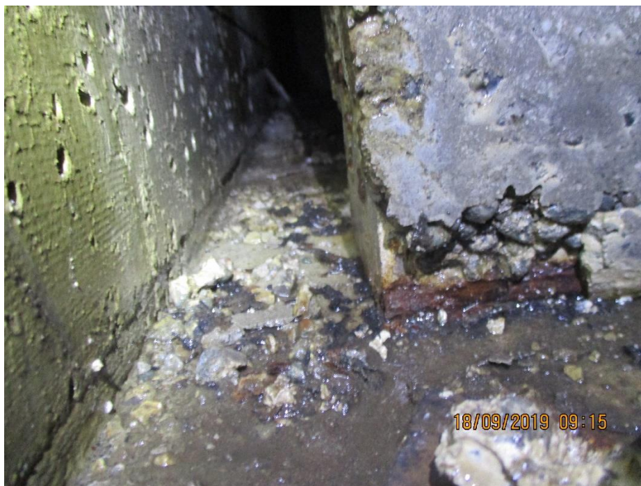
Photo 12 - Spalling of double-tee joist and exposed reinforcing steel
