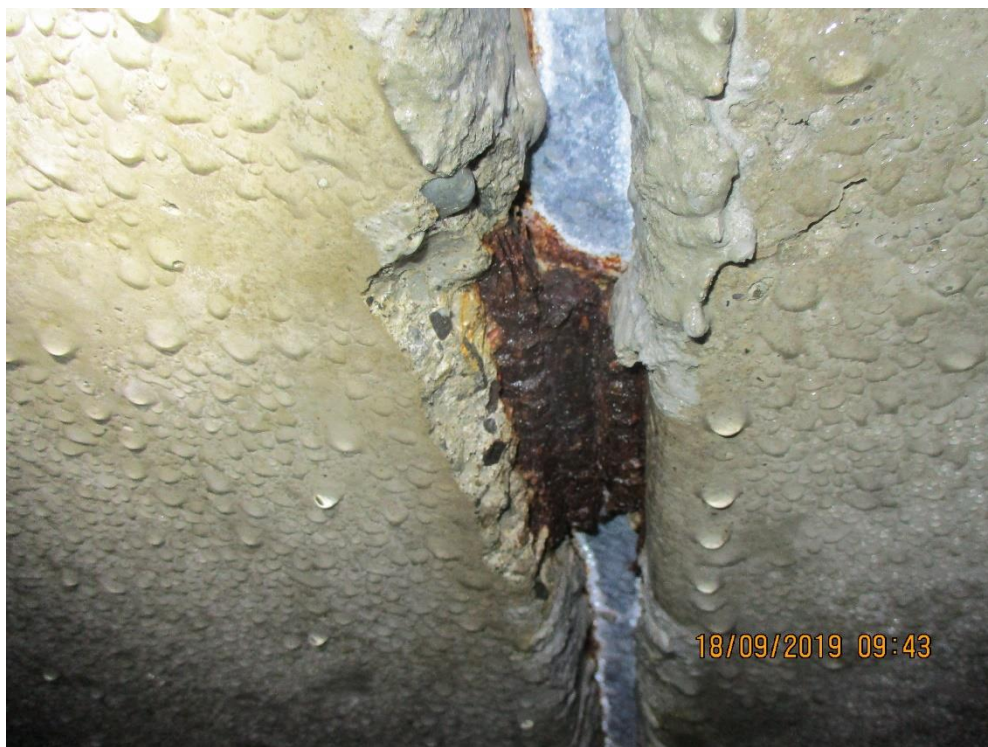
Photo 14 - Corroded steel rebar connection between joists
