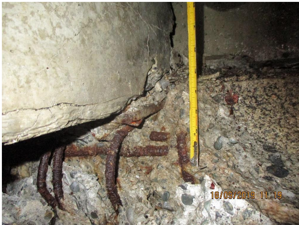
Photo 5 - Concrete girder support at Grid A-8 and 2" settlement
