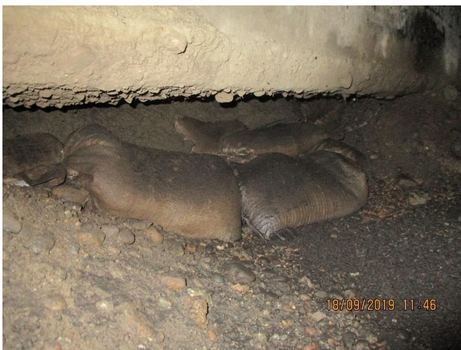
Photo 22 - Undermined reservoir wall located on west side of structure
