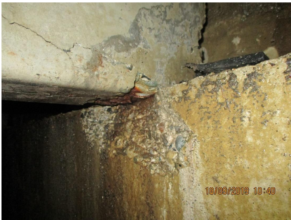
Photo 3 - Spalling of girder and its support (typical condition)
