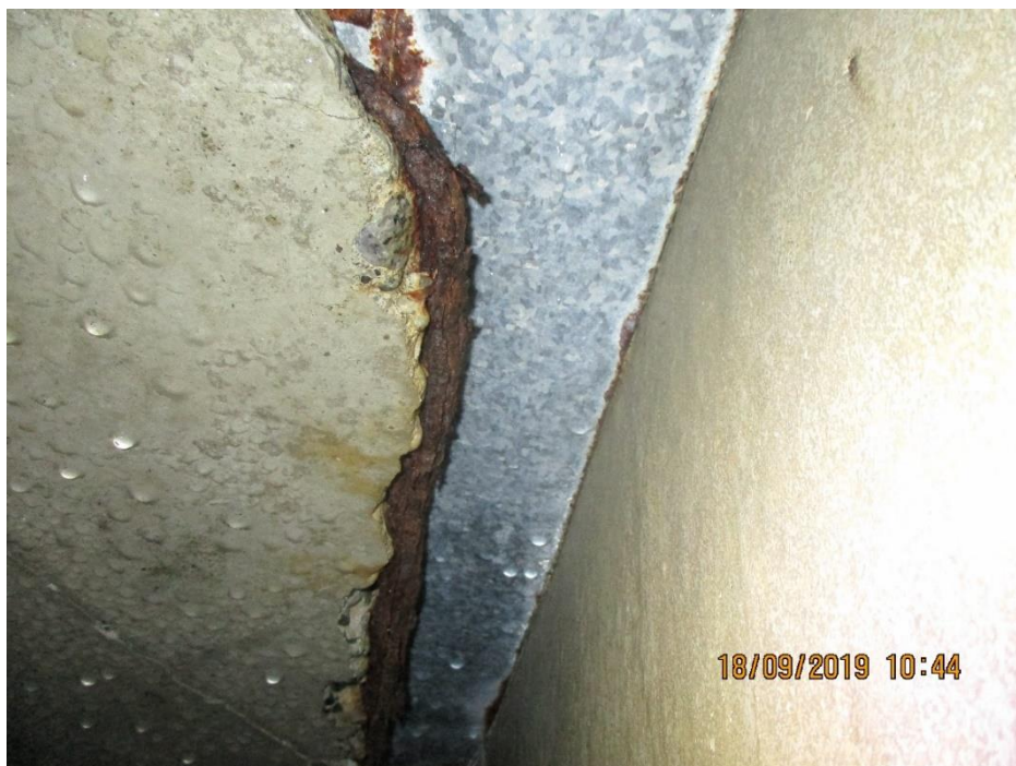
Photo 15 - Corroded double-tee joist flange at "non-bearing" wall support
