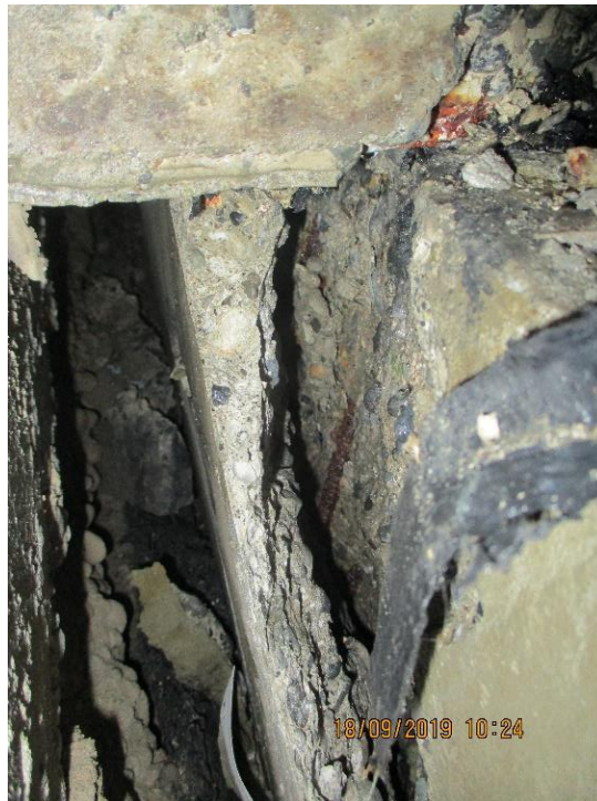
Photo 7 - Spalling at grade beam girder support (typical condition)
