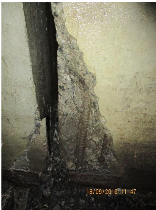
Photo 19 - Spalling and exposed reinforcing steel at exterior wall construction joint at northwest corner
