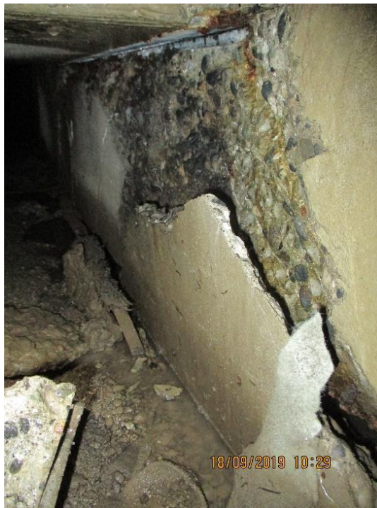
Photo 8 - Spalling at grade beam girder support (typical condition)
