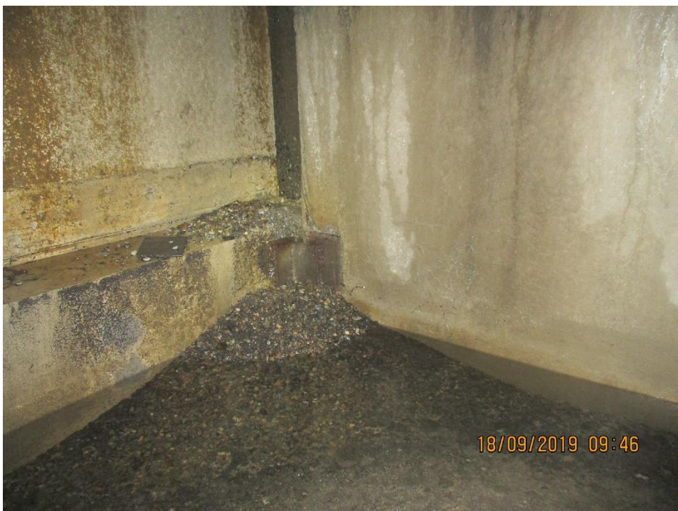
Photo 21 - Standing water at corner crawlspace (typical condition)
