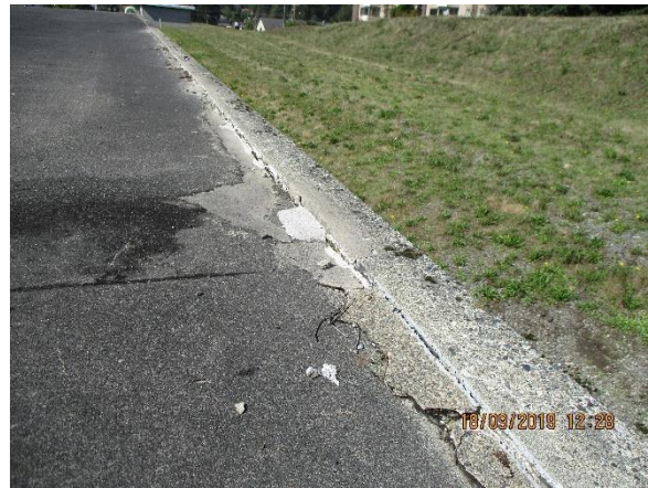
31 - Cracking of topping slab/wall joint at NE
