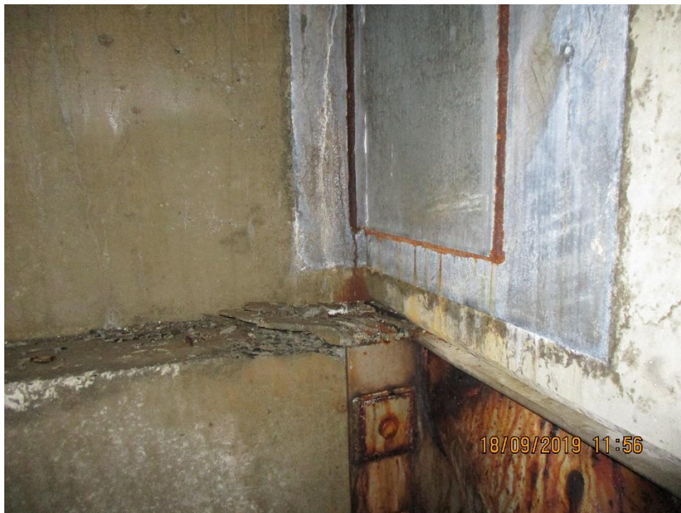
Photo 10 - Spalling of girder at interior support
