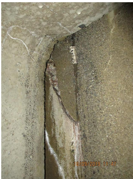
Photo 20 - Spalling and at exterior wall construction joint (same location as previous photo)
