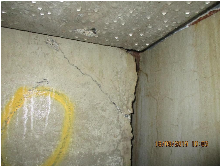
Photo 1 - Spalling at top of girder (typical condition)
