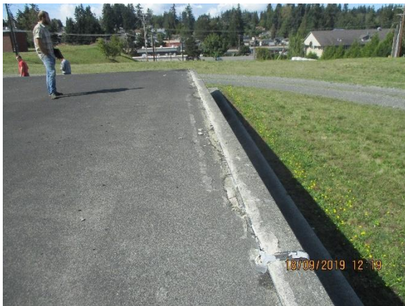
29 - Cracking of topping slab/wall joint at NW corner
