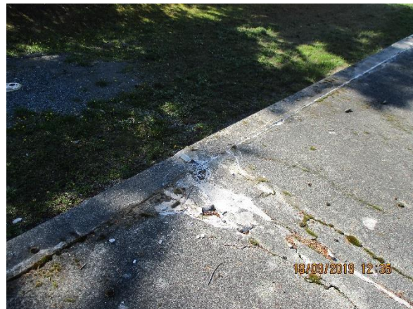
30 - Cracking of topping slab/wall joint at south side
