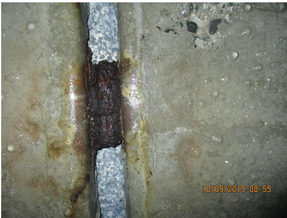
Photo 13 - Corroded steel rebar connection between joists
