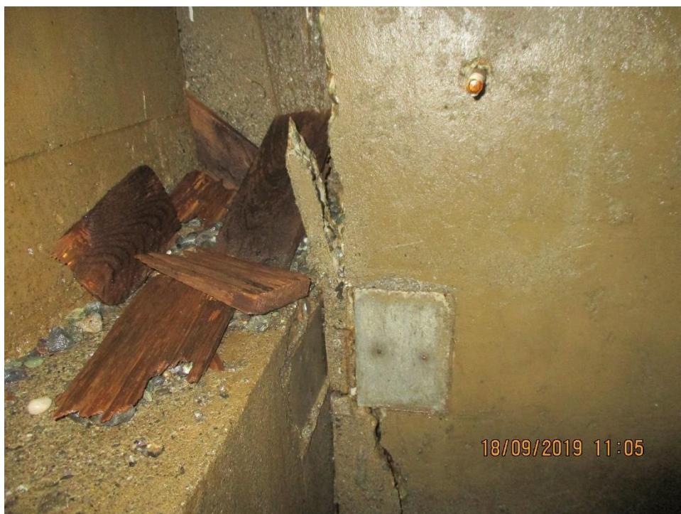
Photo 18 - Spalling around steel connectors at grade beam corner connection
