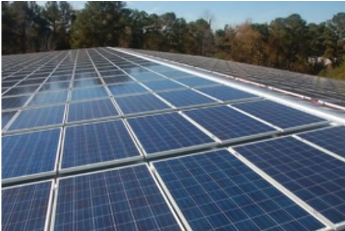
Figure 3: Rooftop Solar with Minimal Spacing
