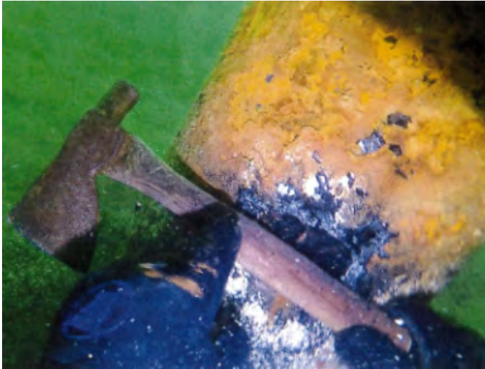
Photo 115A: Pile D, 5" W x 2" H hole
