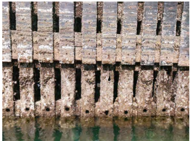
Photo 88: Right wingwall with rot below UHMW sheets
