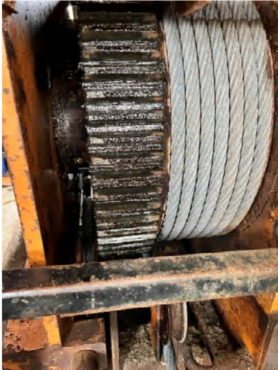
Photo 185: Hoist machine gear and wire rope
