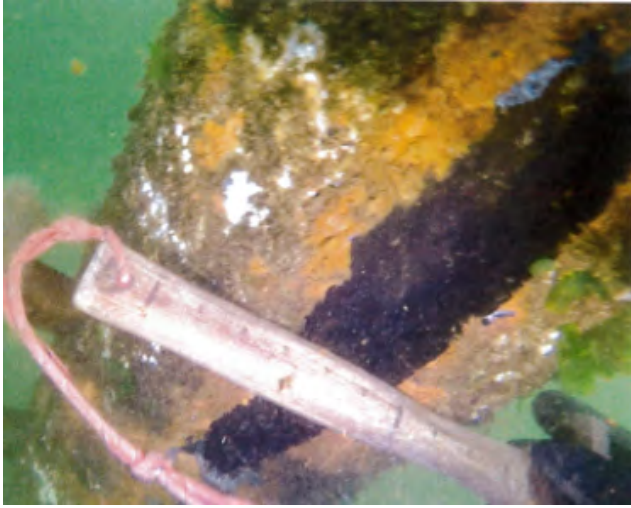
Photo 118: Pile J, 3" W x 18" H hole from mechanical abrasion
