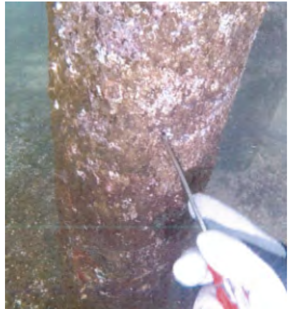
Photo 82: Pile 4A Marine borer entry
