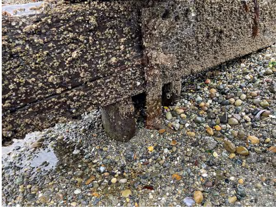
Photo 144: Pile 6A, hollowing around pile cap fastener
