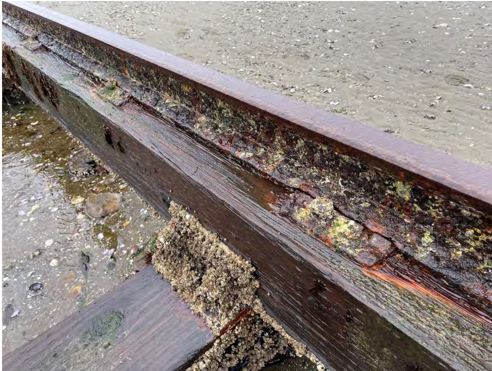
Photo 141: Heavy surface corrosion on rail and pile cap connection bracket
