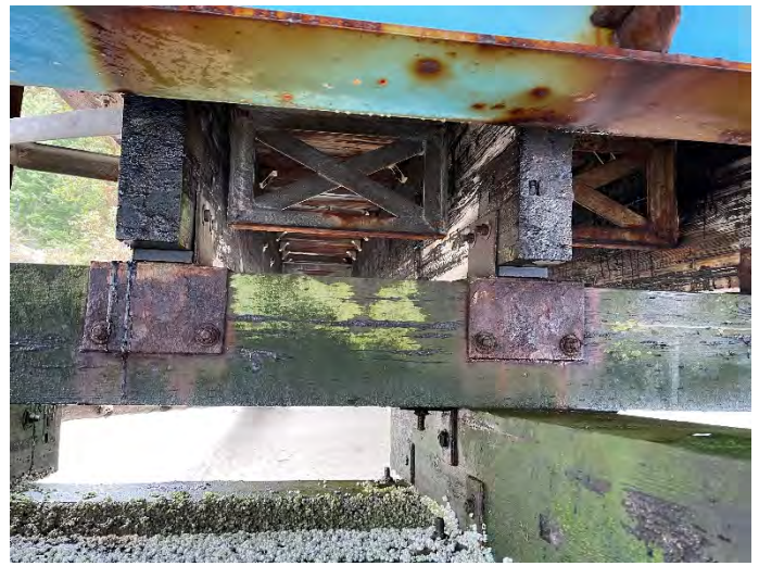
Photo 98: Heavy surface corrosion on girder brackets
