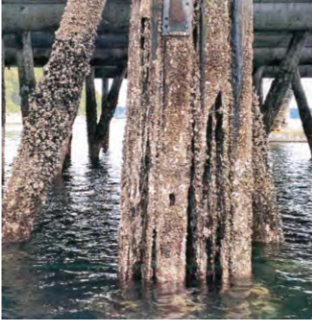
Photo 67: Dolphin D3 with abrasion damage and internal decay
