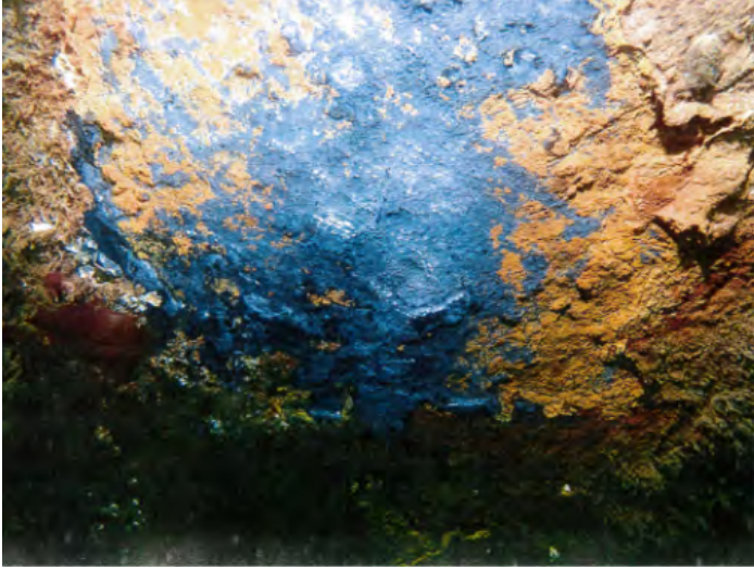
Photo 33: SP3B surface corrosion and section loss
