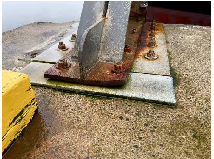
Photo 48: Bent fender with surface corrosion
