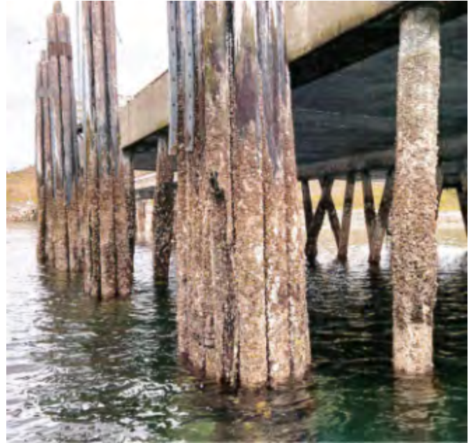
Photo 68: Dolphin D4 with abrasion damage and internal decay
