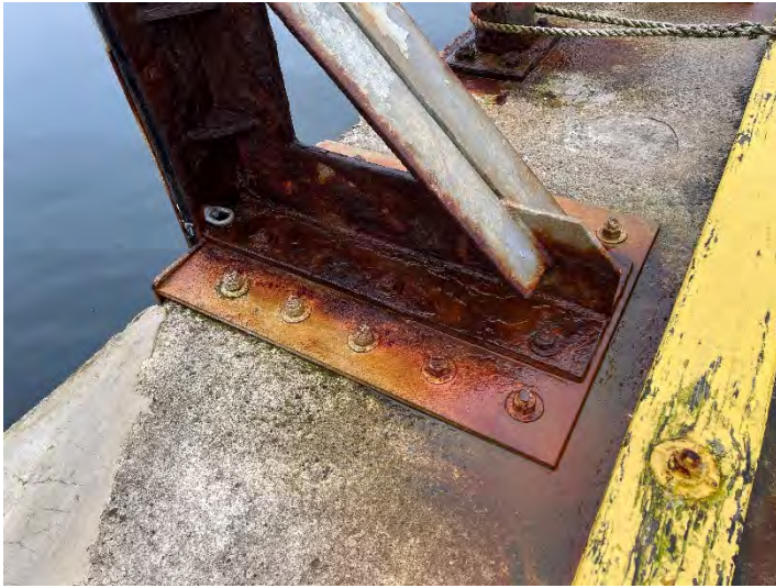
Photo 47: Fender with surface corrosion
