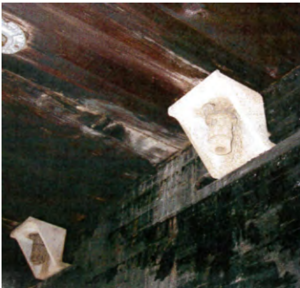
Photo 83: Loose timber deck hold down bolts
