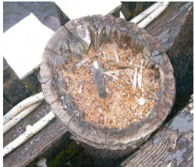
Photo 84: Typical wingwall pile with top rot
