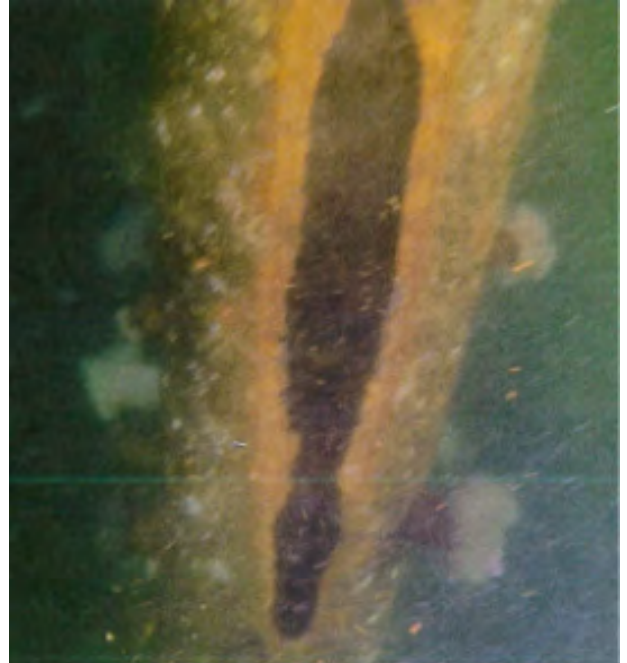
Photo 114: Pile D, 4" W x 36" H hole from mechanical abrasion
