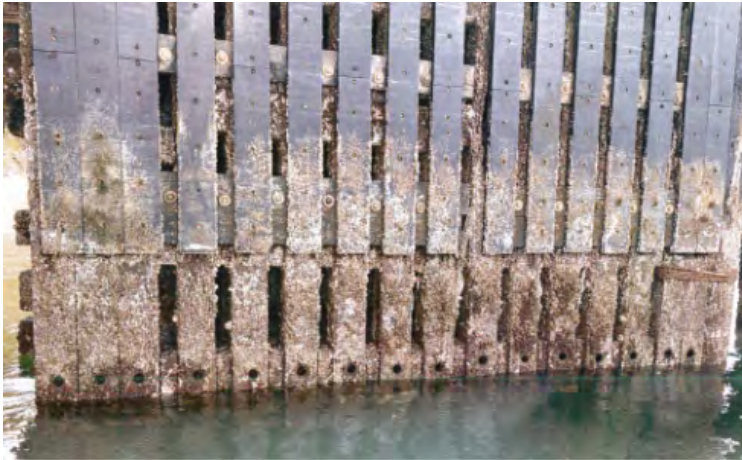
Photo 85: Left wingwall with rot below UHMW sheets
