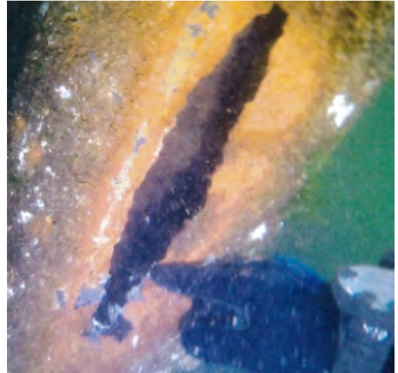
Photo 115B: Pile E, 2" W x 18" H hole from mechanical abrasion
