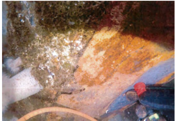
Photo 36: SP2-A heavy corrosion and section loss
