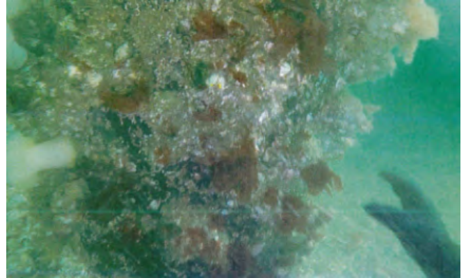
Photo 92: Pile 3A, typical conditions of other piles
