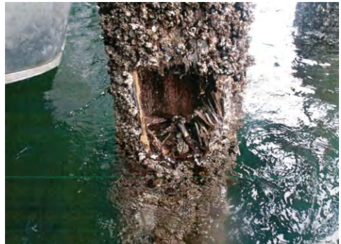
Photo 9: Pile 8.9A Rot cavity (2017) 9"W x 16"H x 8"D
