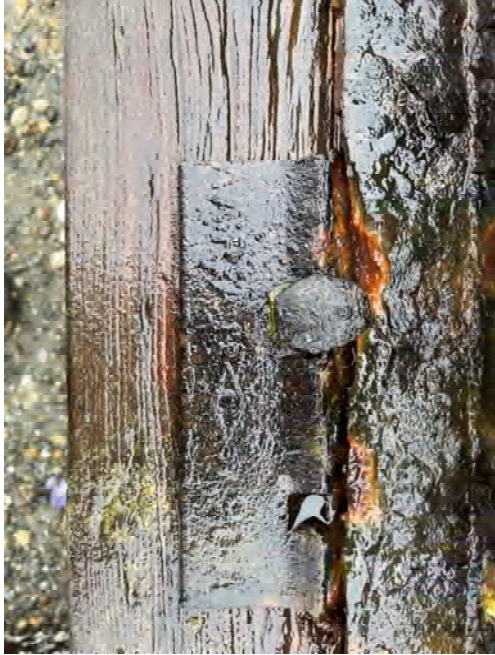
Photo 169: Rail clip and rail near bulkhead burning up
