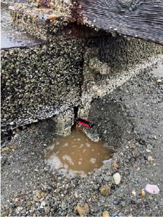
Photo 146: Pile 10B, hollowing around pile cap fastener
