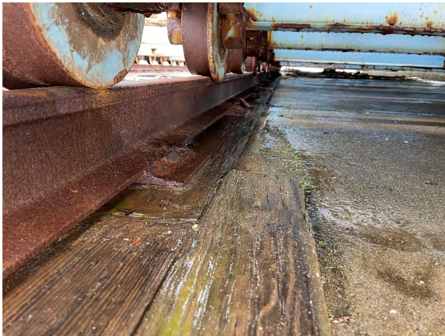
Photo 127 : Rail pitting and surface corrosion North of bulkhead
