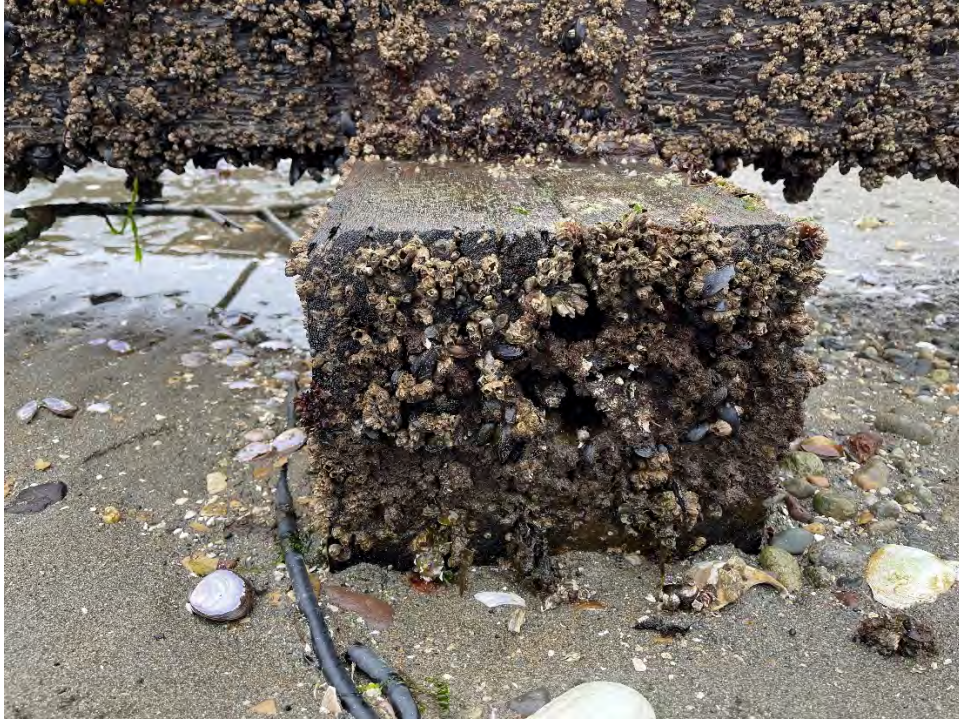
Photo 142: 15 th pile cap with early stages of hollowing
