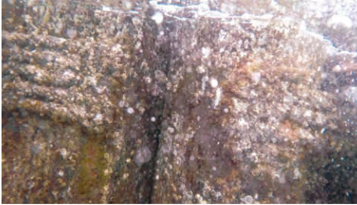
Photo 91: Left wingwall end dolphin lower wraps broken
