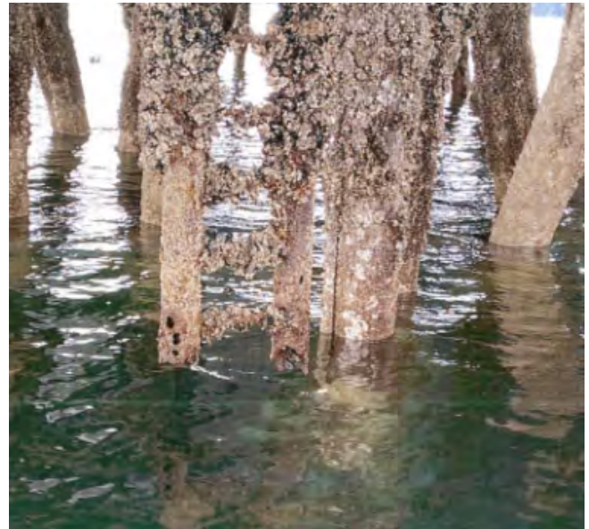
Photo 70: Boat lift access ladder has corroded off in lower intertidal zone.
