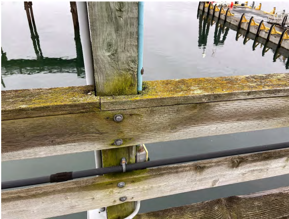
Photo 20: Wooden guard rail with heavy green moss algae
