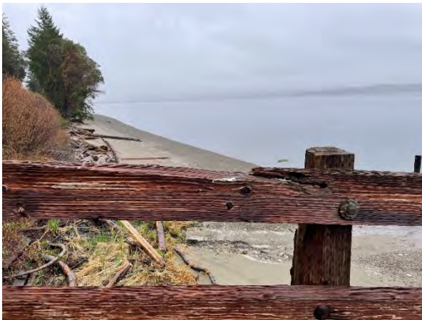
Photo 101: Timber guard rail splitting
