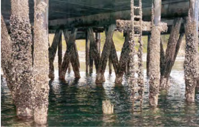
Photo 63: Pile F10 broken, South ladder is unsecured
