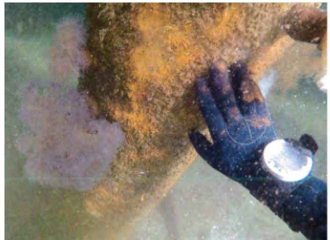
Photo 125: Typical pile condition underwater, 25%-50% coating failure and surface corrosion
