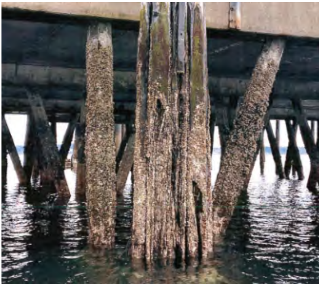
Photo 69: Dolphin D1 with abrasion damage and internal decay
