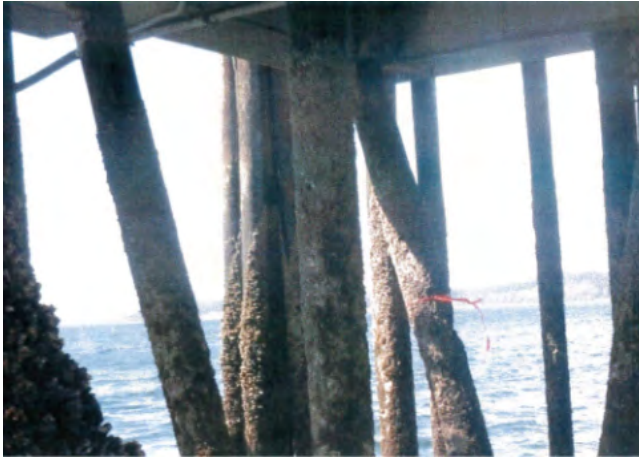
Photo 10: Pile 8.9A Rot cavity (2021) 12"W x 21"H x 12"D
