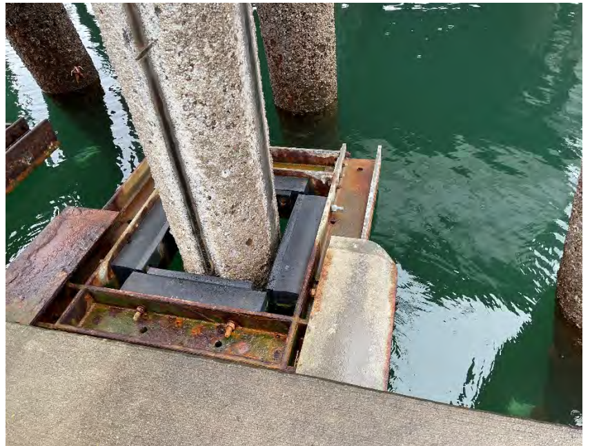
Photo 30: Pile collar with bent angle from batter pile
