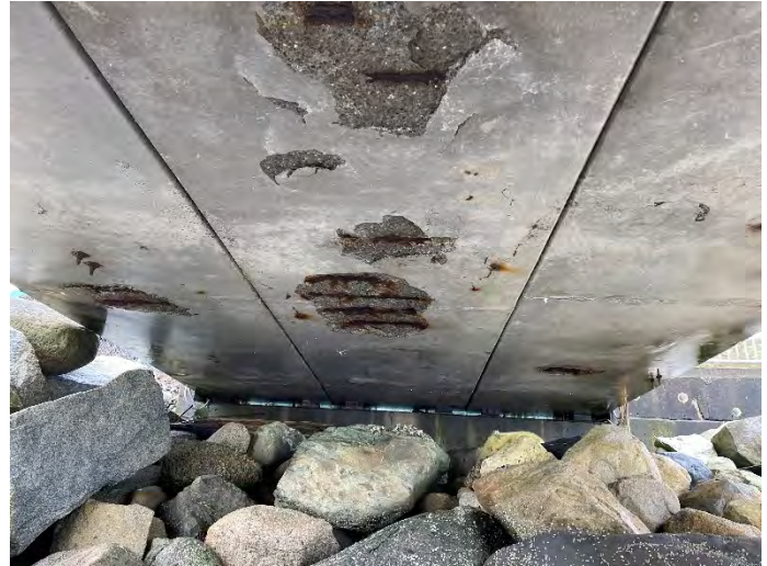
Photo 72: Concrete spalling below trestle
