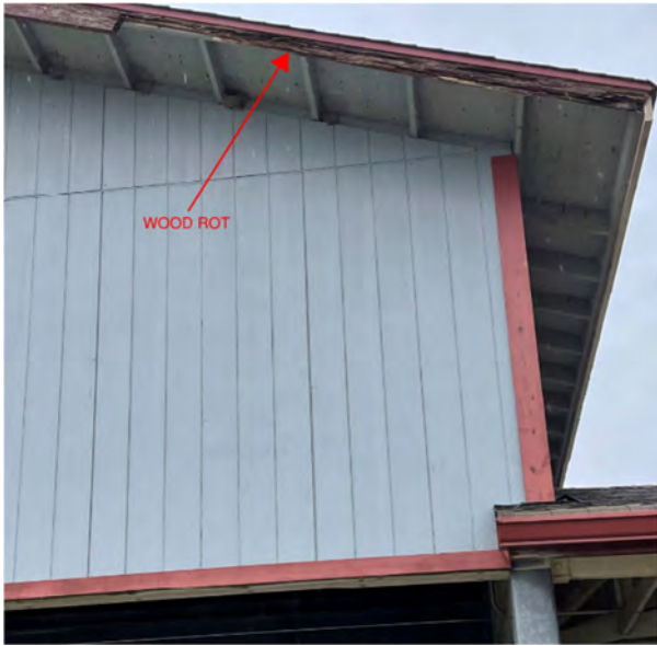
Photo 79: Wood rot on Fascia board
