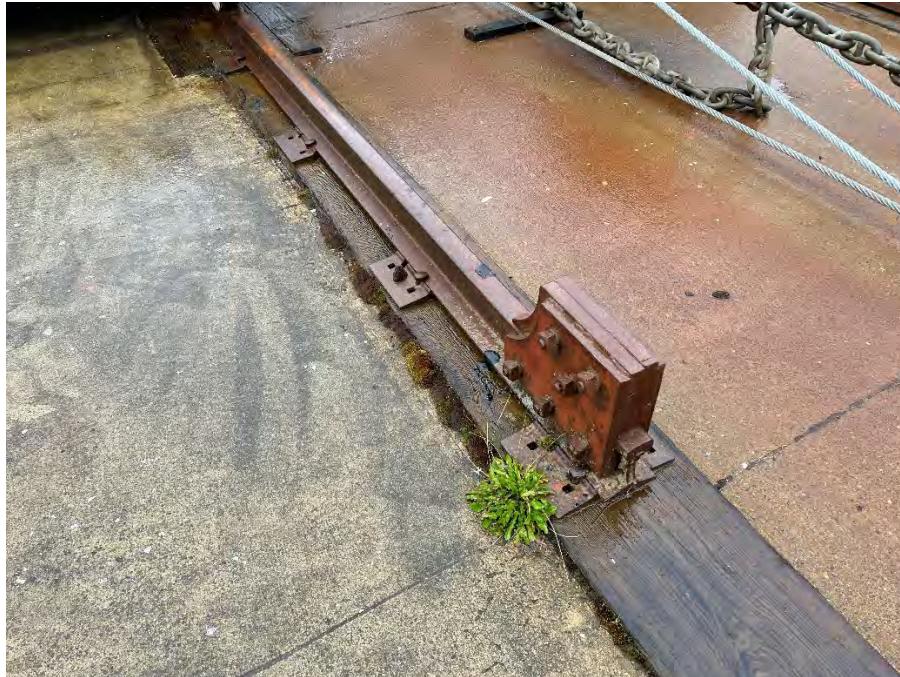
Photo 126 : Surface corrosion on rail North of bulkhead
