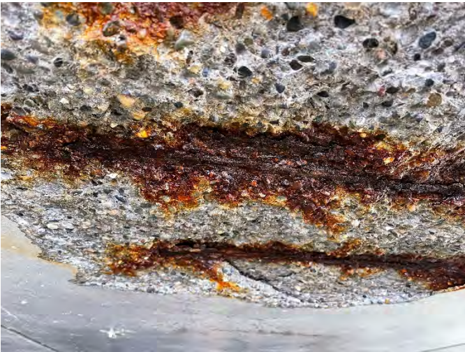
Photo 73: Exposed reinforcement from concrete spalling
