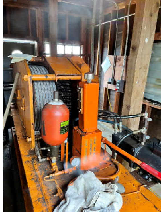
Photo 186: Hoist machine gear and wire rope
