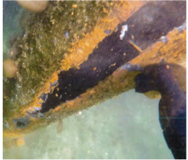
Photo 112: Pile P, 3 ft vertical hole from mechanical abrasion
