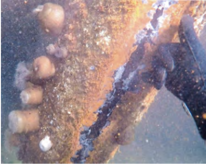
Photo 111: Pile O, 18" H x 4" W hole from mechanical abrasion
