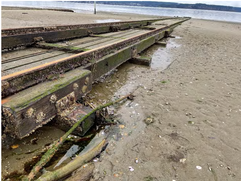
Photo 151: Timber rail splice beam with heavy marine growth
