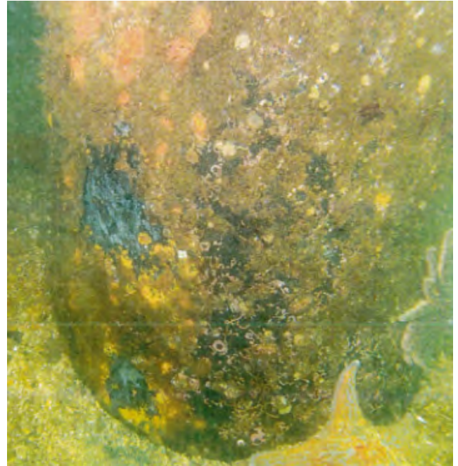
Photo 42: SP4-B typical coating failure and surface corrosion
