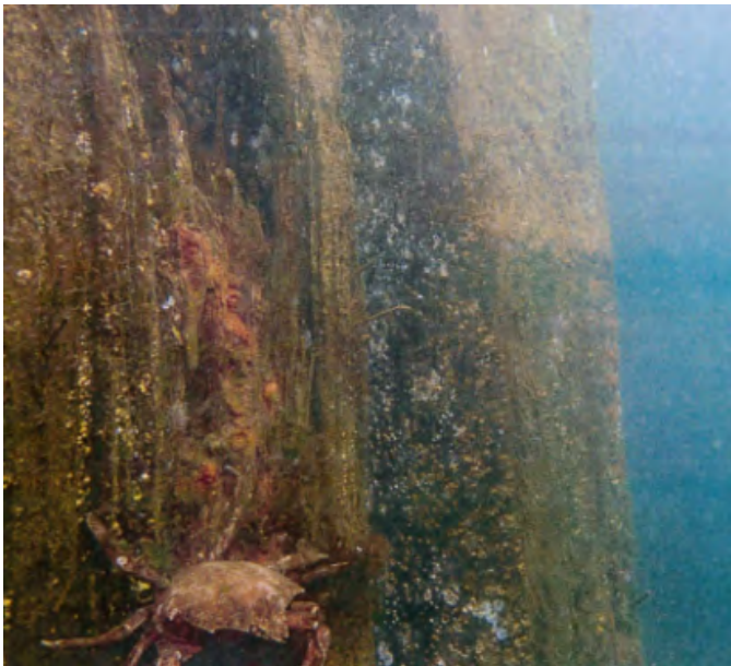
Photo 65: Dolphin D1, mechanical damage, and MBE holes
