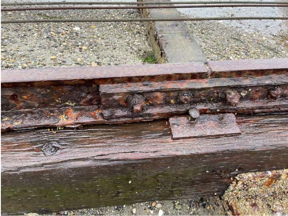
Photo 138: Rail splice plate with heavy surface corrosion
