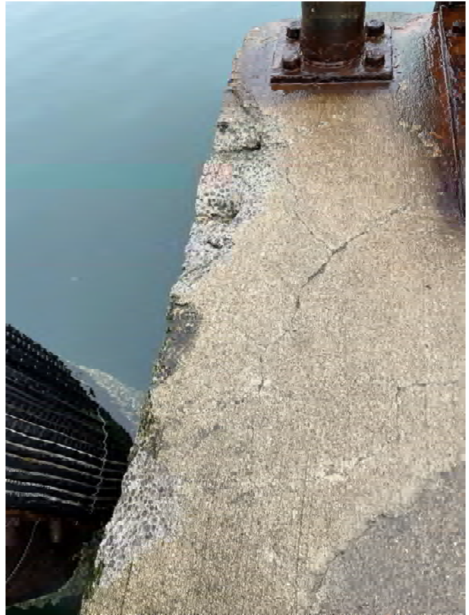
Photo 52: Concrete spalling along edge of float
