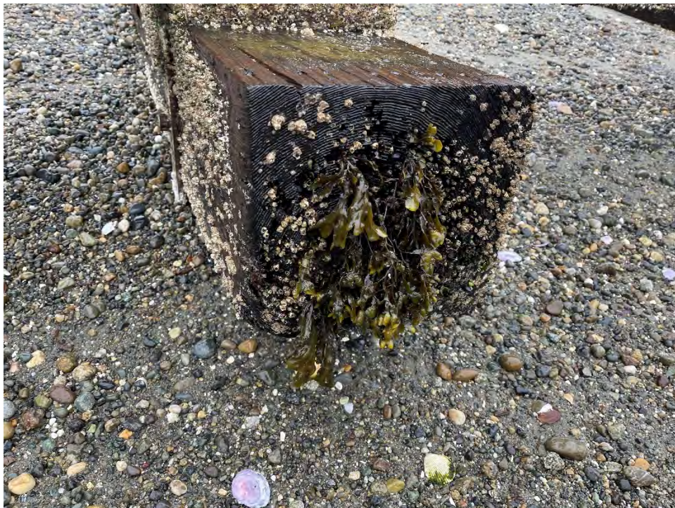
Photo 143: 17 th pile cap with early stages of hollowing
