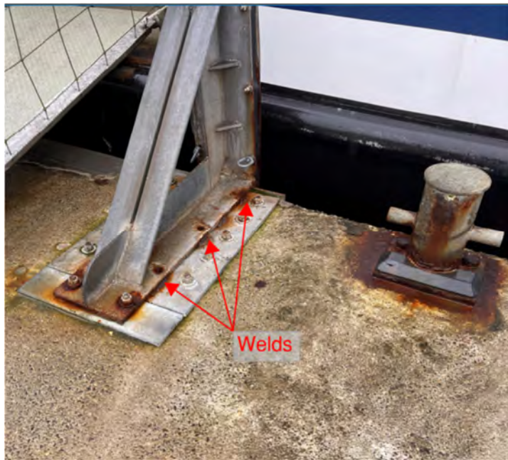
Photo 49: Missing fasteners on fender, secured by welds
