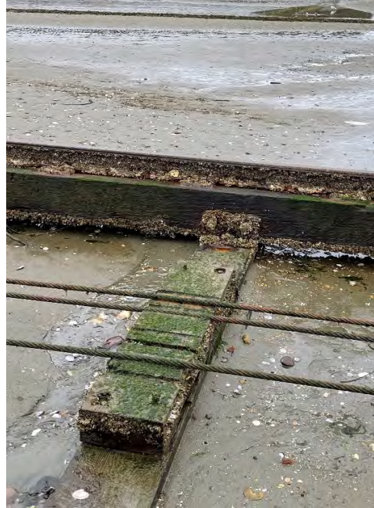
Photo 147: Wire rope wearing on pile cap rub beam
