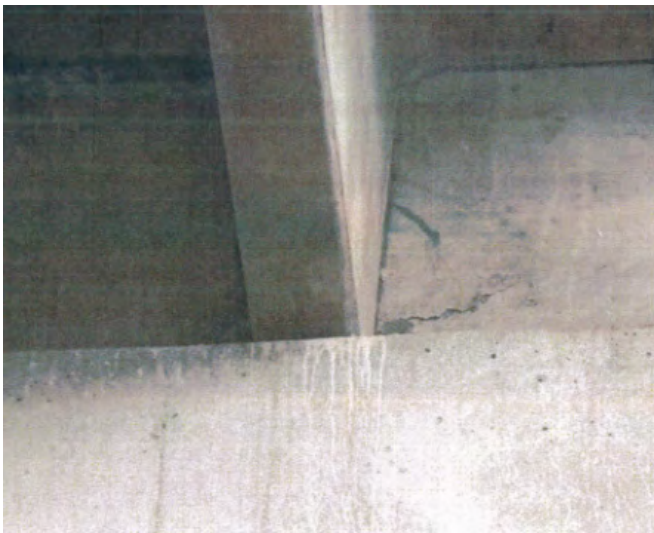
Photo 106: Pier 7 end diaphragm has delamination at the left web of Span 7
