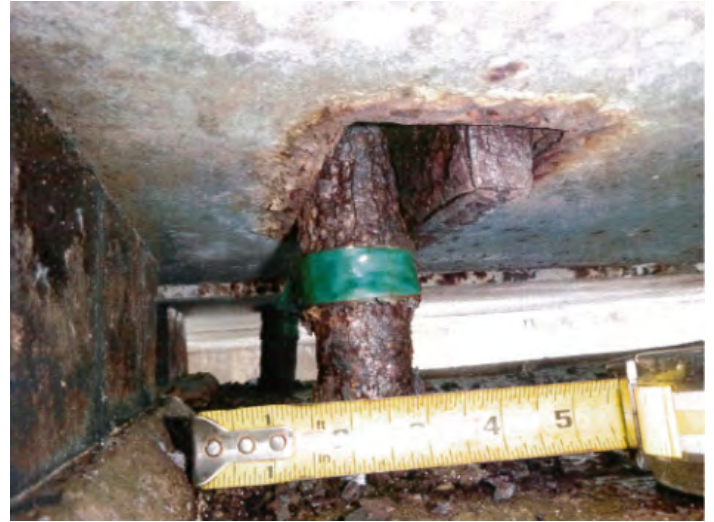
Photo 64: Deck panel 7B hold down bolt is necked down to 1.1875" at pier 7
