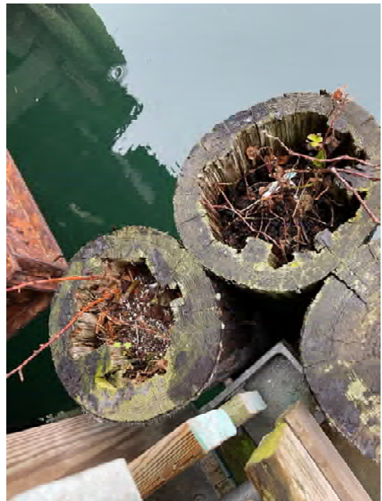
Photo 78: Piles F2A,B,C rot at top of piles
