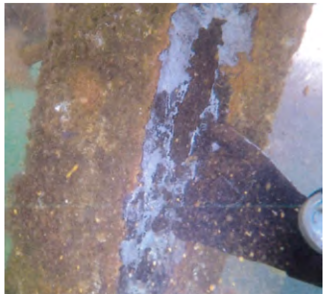
Photo 111: Pile J, 12" H x 2.5" W hole from mechanical abrasion
