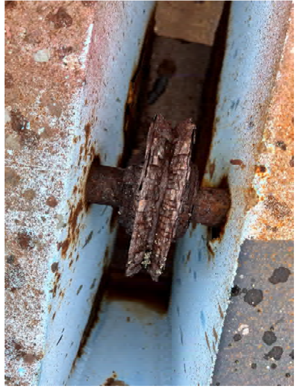
Photo 192: Bilge block pulley
