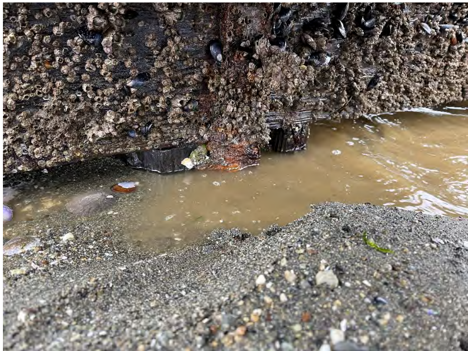
Photo 145: Pile 9A, hollowing around pile cap fastener
