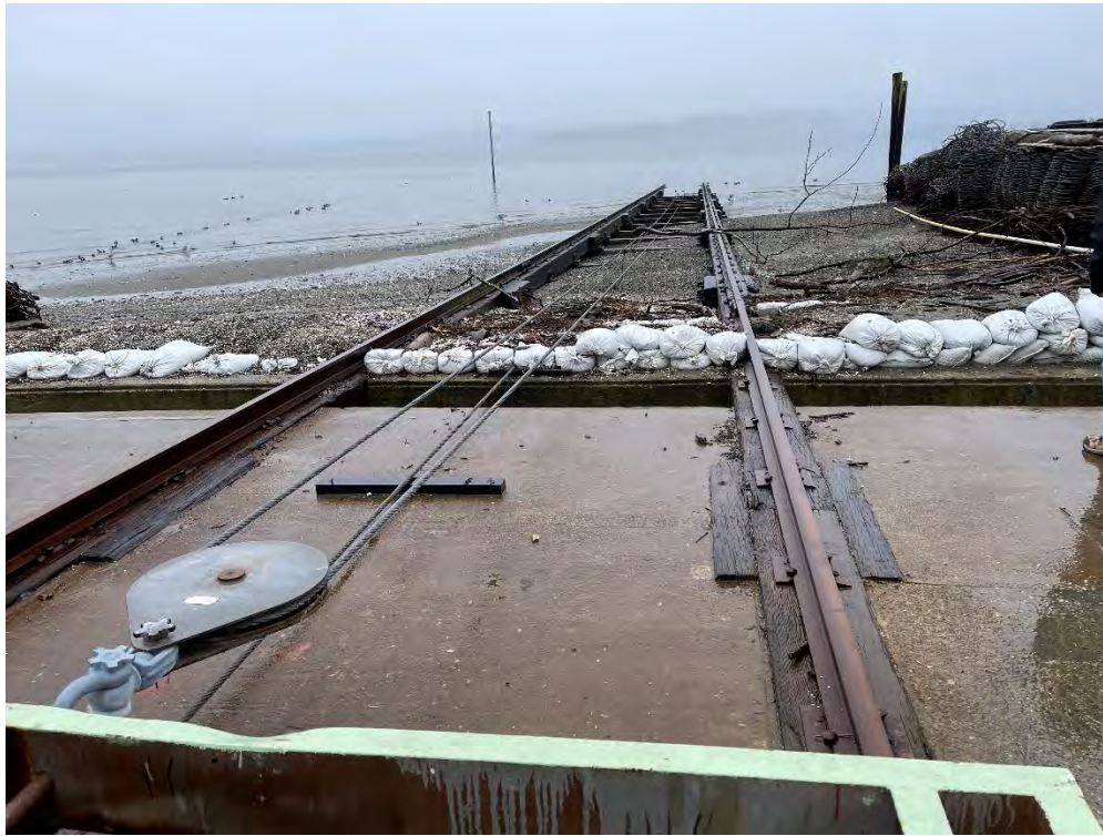
Photo 130: Rail system looking South
