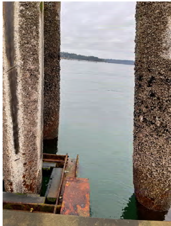
Photo 28: Pile collar with bent angle from batter pile
