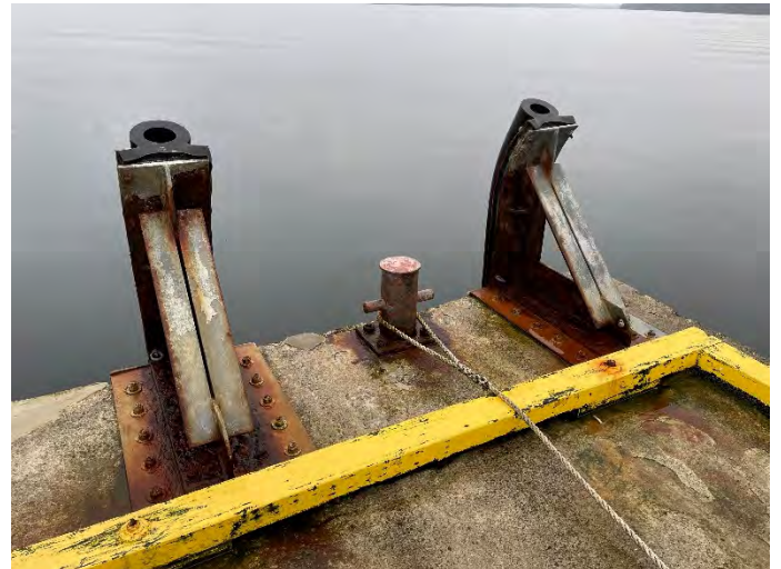
Photo 50: Mooring cleat with surface corrosion
