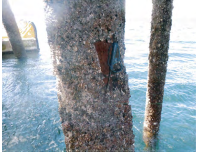
Photo 11: Pile 8.9A Rot cavity (2019)
