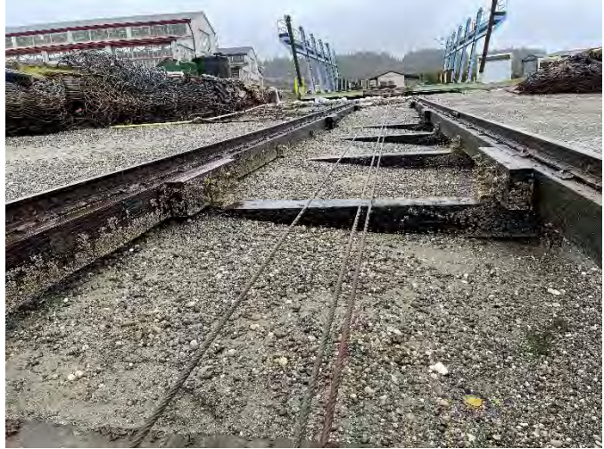
Photo 170: Rail system looking North
