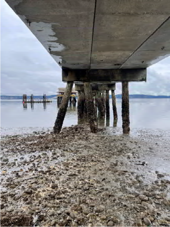
Photo 71: Concrete spalling below trestle
