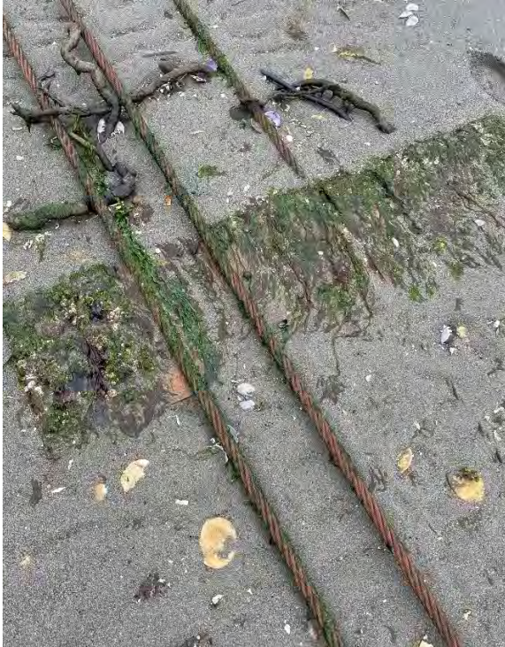
Photo 148: Wire rope wearing on pile cap rub beam
