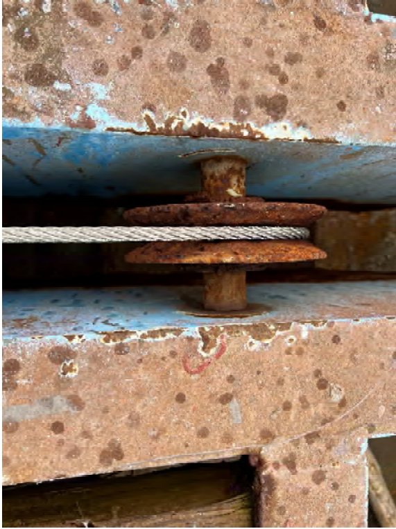
Photo 191: Bilge block pulley
