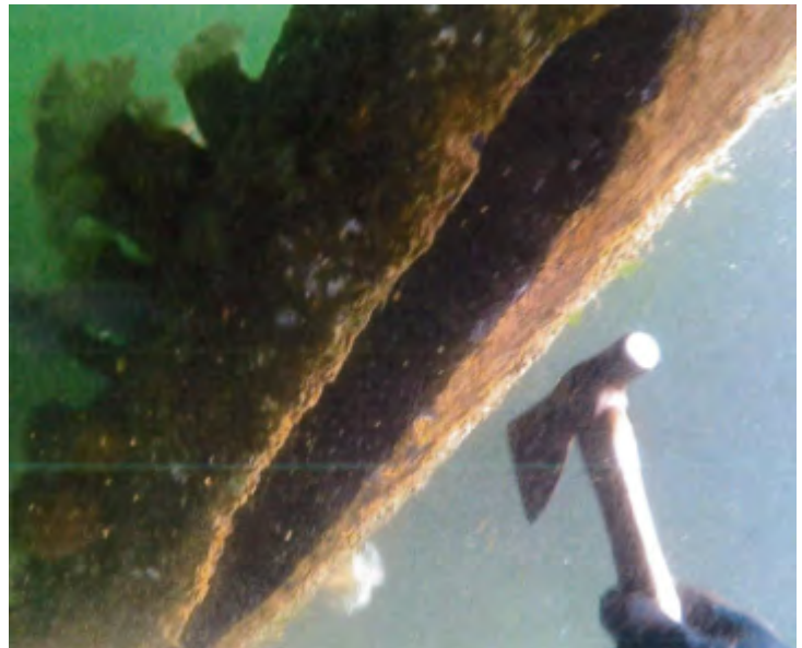
Photo 121: Pile P, 5" W x 54" H hole from mechanical abrasion
