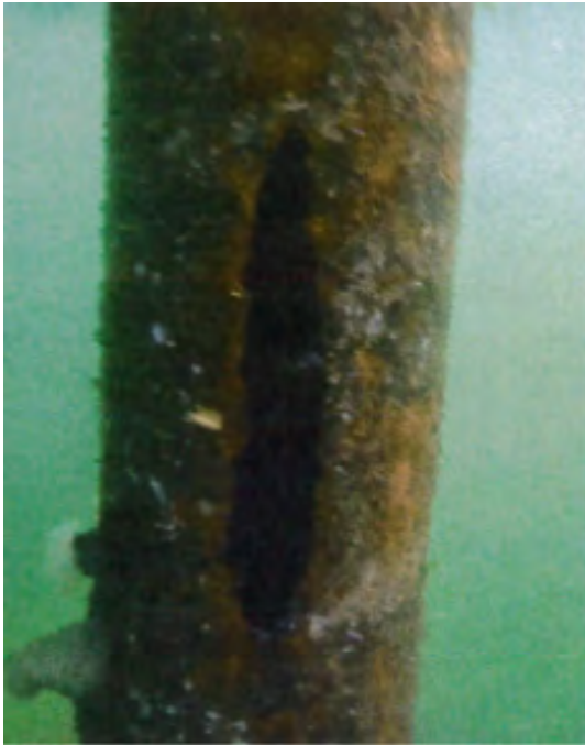
Photo 120: Pile O, 4" W x 24" H hole from mechanical abrasion
