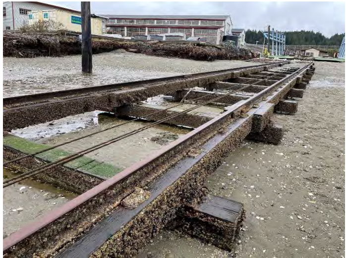
Photo 172: Rail system looking North
