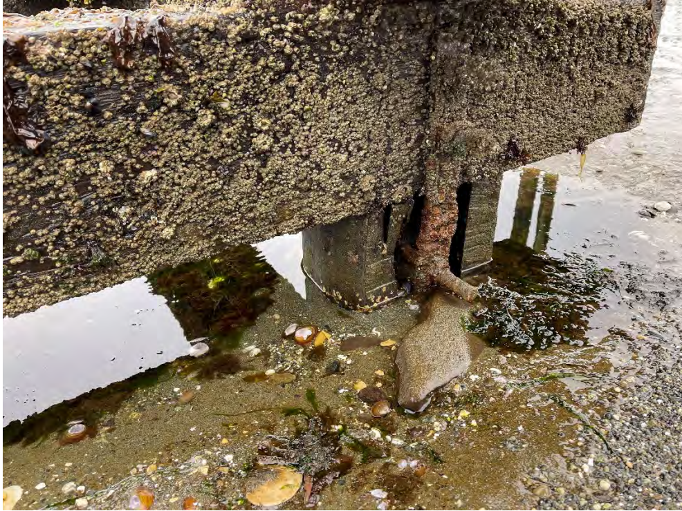
Photo 153: Pile 12A, hollowing around pile cap fastener
