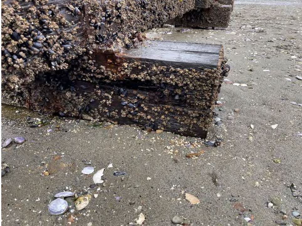
Photo 150: 16 th pile cap with hollowing
