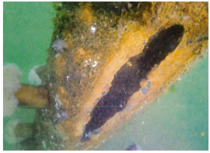
Photo 119: Pile L, 3" W x 24" H hole from mechanical abrasion
