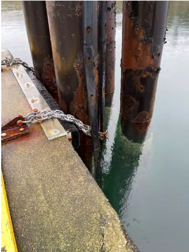
Photo 53: Chain rubbing on pile, UHMW rub rails failing
