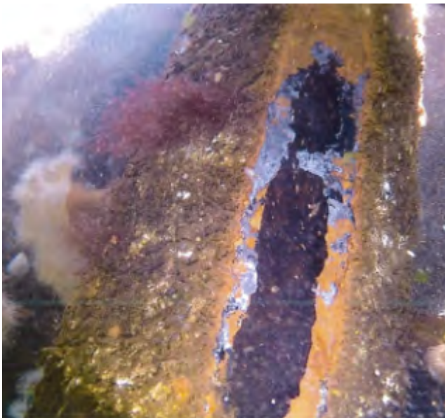
Photo 110: Pile A, 18" H x 4" W hole from mechanical abrasion
