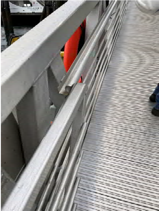
Photo 21: Loading ramp handrail with sharp edge
