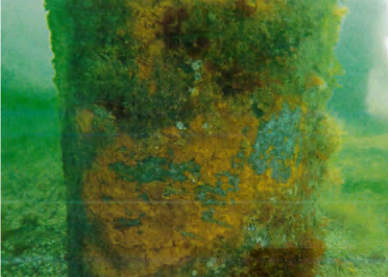
Photo 34: SP4 coating failure and surface corrosion
