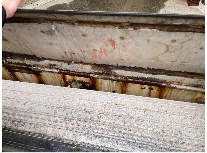
Photo 60: Surface corrosion on connections between floats
