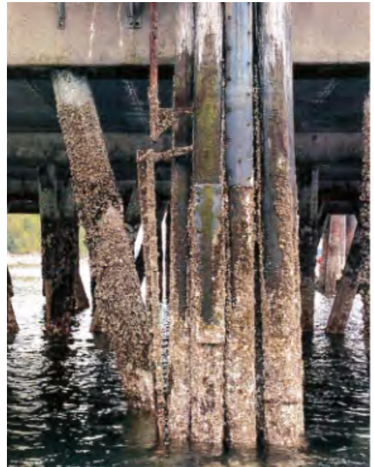
Photo 66: Dolphin D2 with abrasion damage, ladder detached
