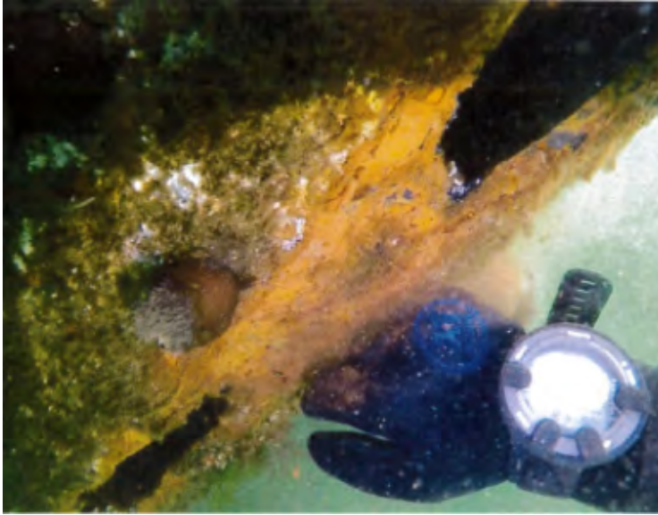
Photo 122: Pile V, 4" W x 24" H hole and 3" W x 14" H hole from mechanical abrasion
