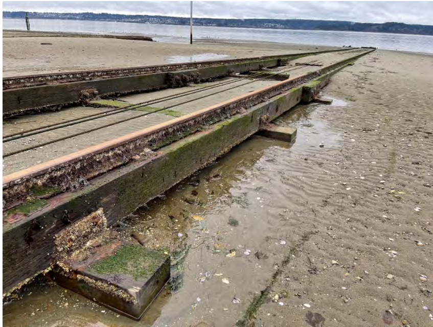
Photo 173: Rail system looking South
