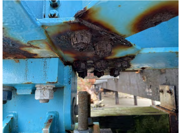
Photo 100: Heavily corroded and delaminating nuts
