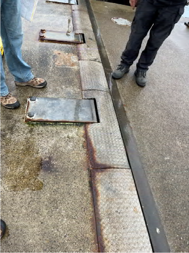
Photo 59: Surface corrosion on cover plate
