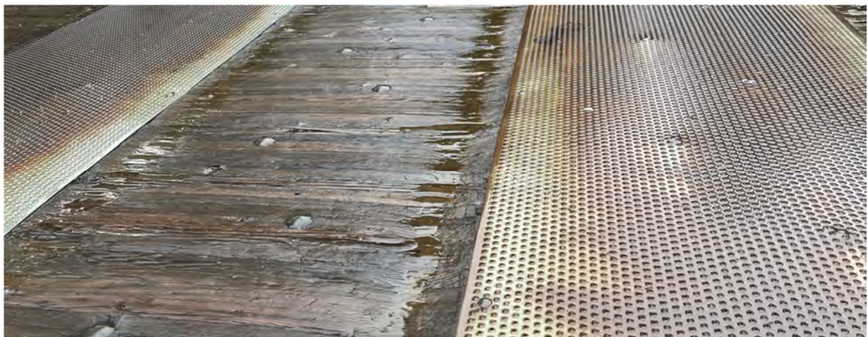
Photo 103: Timber deck is rutting
