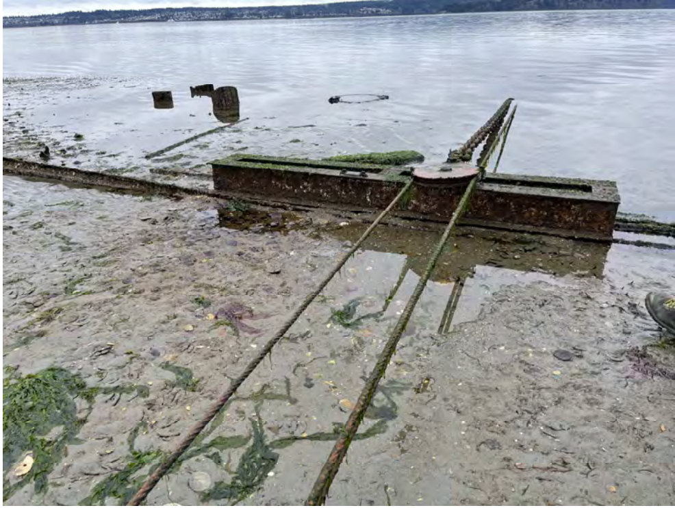
Photo 154: Anchor system at Southern end of track
