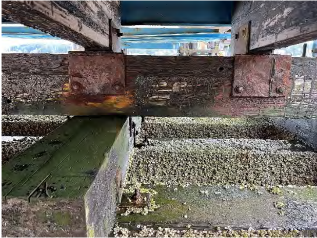
Photo 99: Heavily corroded and delaminating girder brackets
