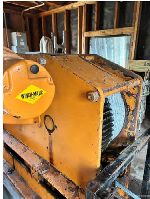
Photo 184: Hoist machine electric motor
