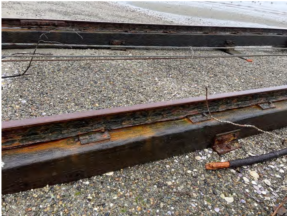
Photo 137: Heavy surface corrosion on rails and rail clips
