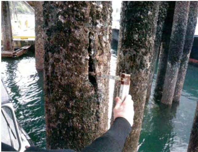
Photo 8: Pile 8.9A Rot cavity (2013) 6"W x 12"H x 6"D
