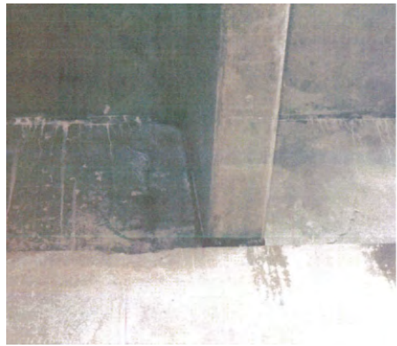
Photo 105: Pier 2 end diaphragm has delamination on the right web of Span 1
