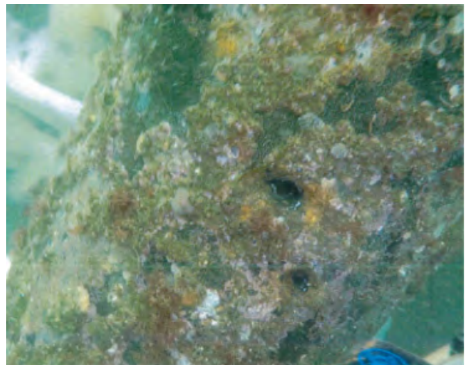
Photo 38: SP3-C holed through pitting
