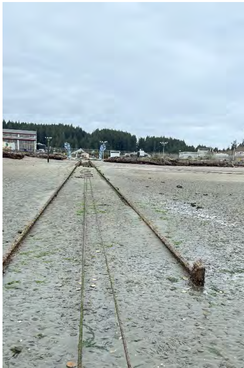
Photo 171: Buried members on Southern section of rail system
