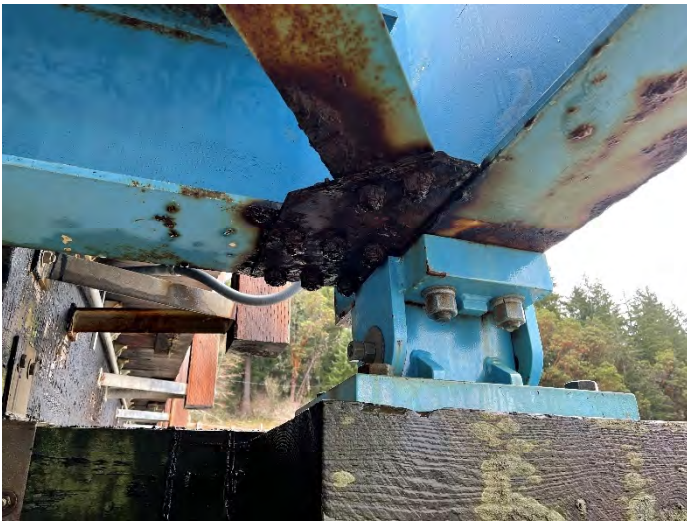
Photo 97: Heavy surface corrosion on fasteners
