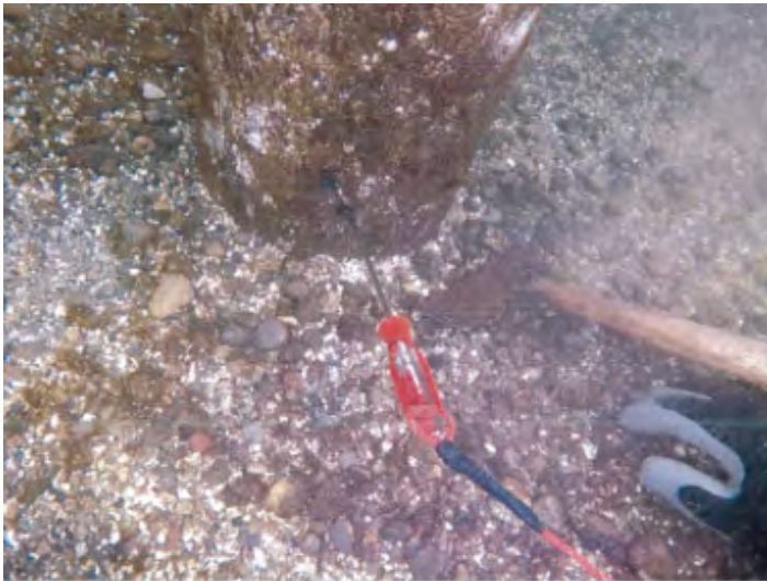
Photo 81: Pile 2C Marine borer entry
