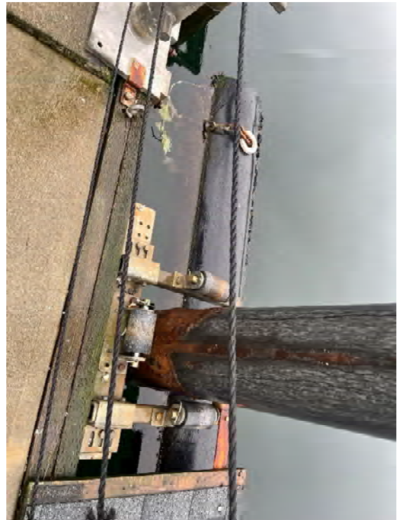
Photo 107: Panels E and F are uneven up to 1"
