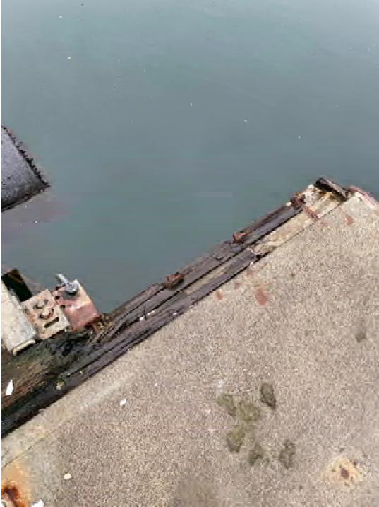
Photo 108: Near Spud Pile A, timber waler is broken and corroding fasteners
