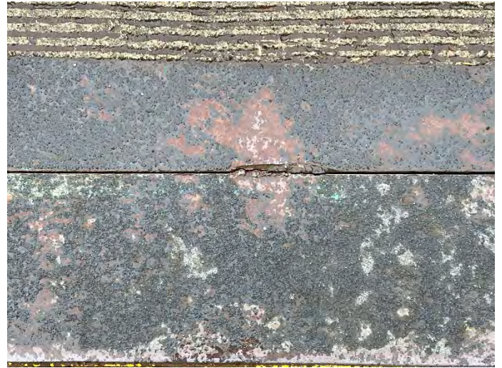
Photo 19: Steel sliding plate stitch welds breaking
