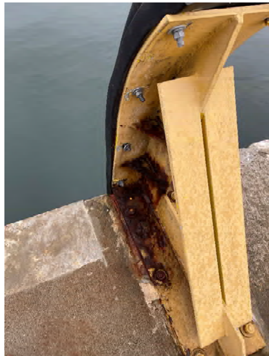
Photo 24: Fender with surface corrosion
