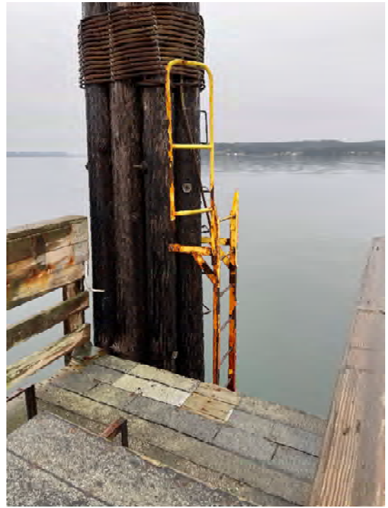
Photo 76: Dolphin ladder broken
