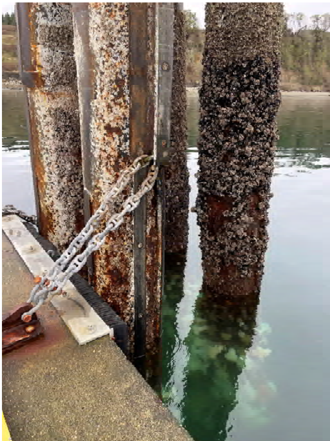
Photo 57: SP3 chain catching on UHMW rub rails
